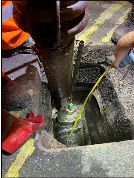
Inspection of the surface water drainage penstock at Fen Lane, Beccles in July 2021.
