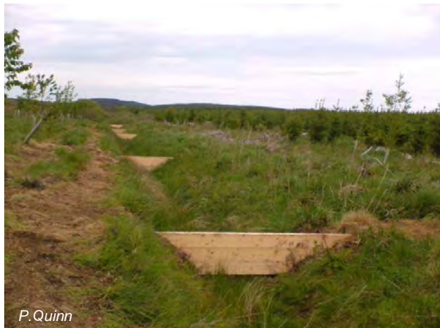
Dams across agricultural field drains to back water up and slow the flow. These are built raised from the bed to allow low flows to pass under the dam and backing water up in higher flows.
