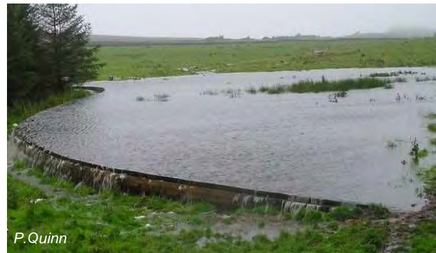
Offline storage area created using leaky timber bund to enable slow release of flow back to the watercourse.
