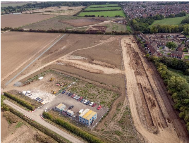
Photo: The Castlehill site, showing the site compound and the realigned Sutton Cross Drain (right side), taken during the summer months.
