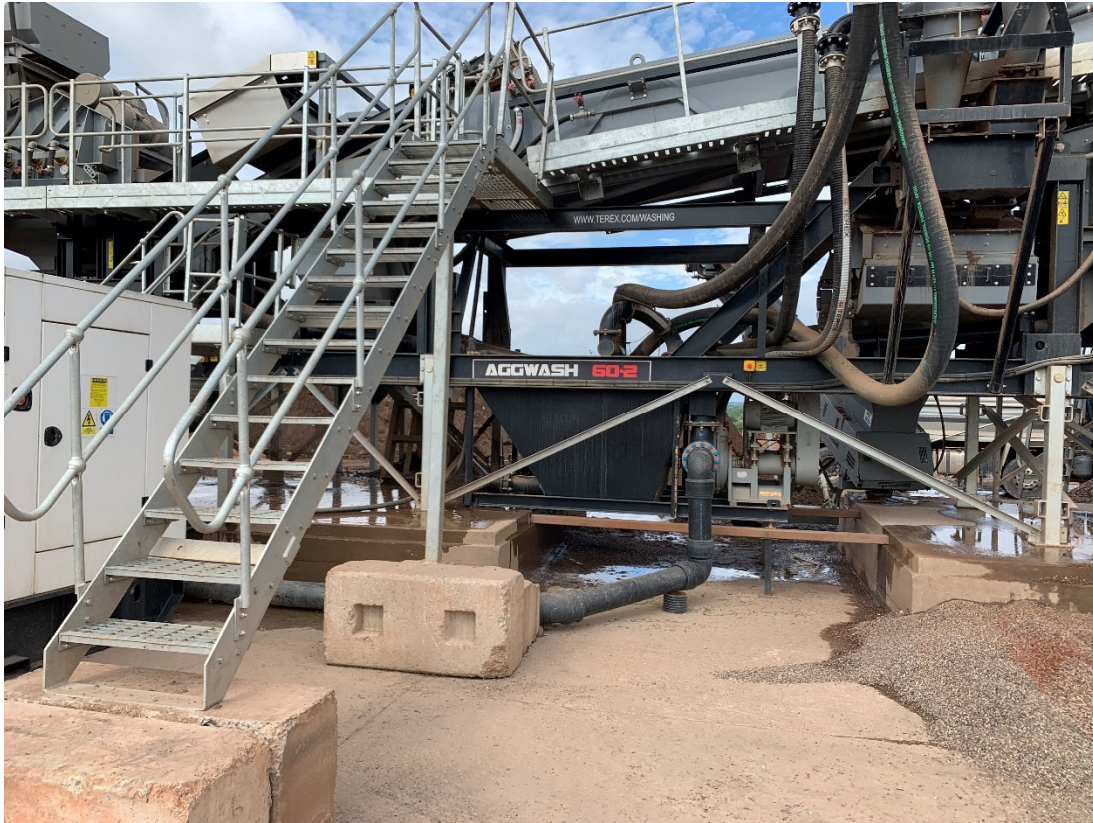
Figure 2.2. Agg Wash Plant
