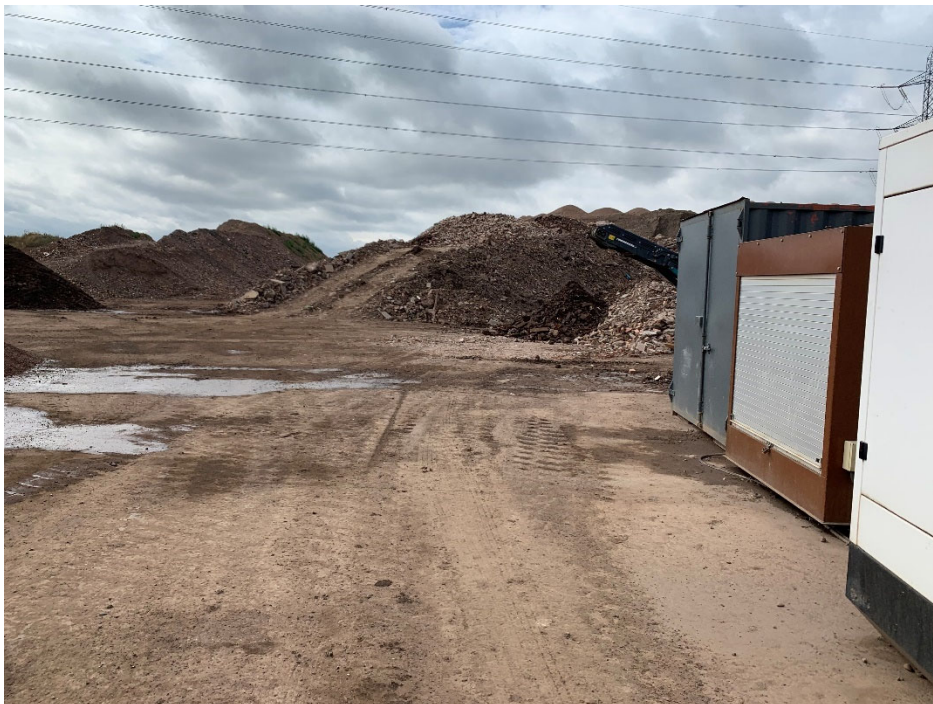
Figure 2.3 Screener and Power for Agg Wash Plant
