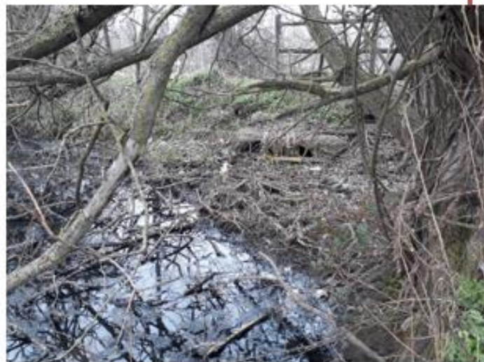
Twin Culvert at Stubbers Green Road, flow into "The Swag". View Northeast.
