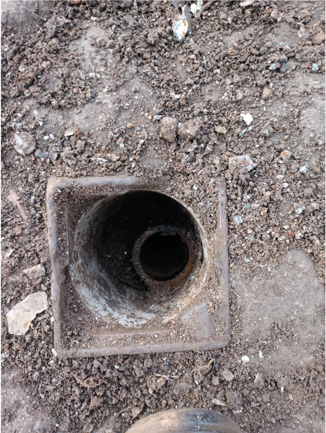
Photograph 2: Photo of BH101 with no steel protective lid
