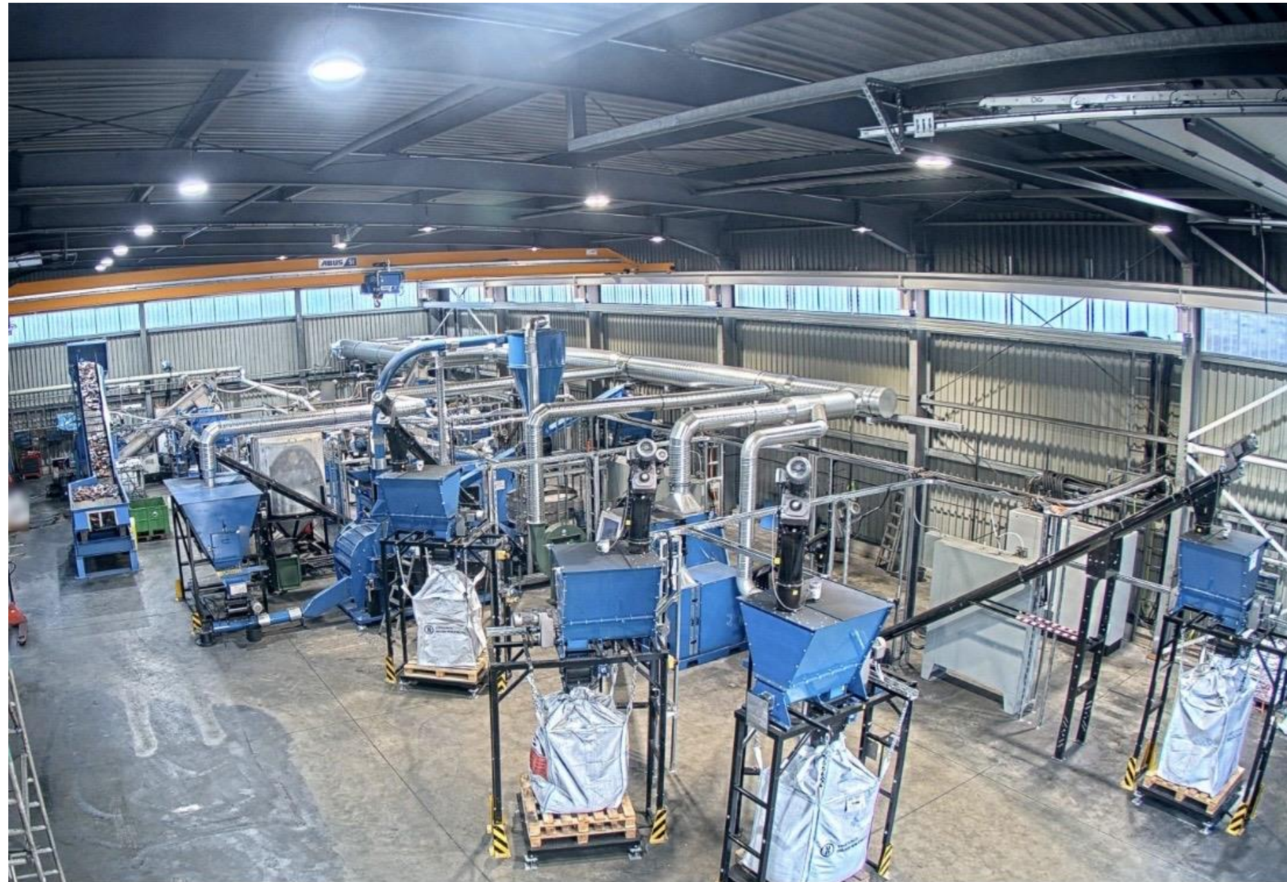
Overview picture from Germany currently commissioning the plant.
