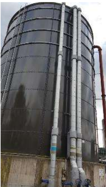
Photo 2: Screened sludge tank
