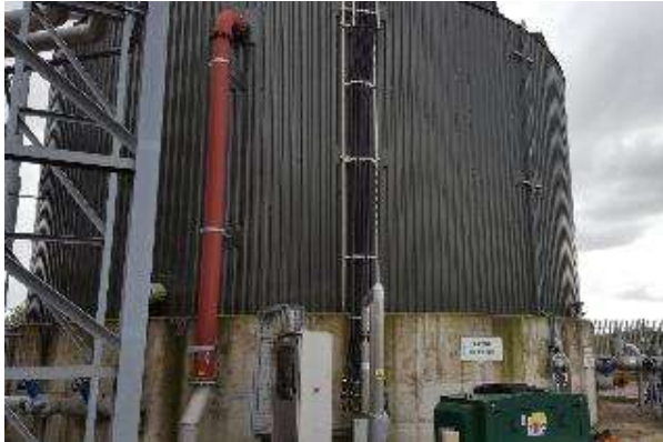
Photo 7: Digested sludge tank
