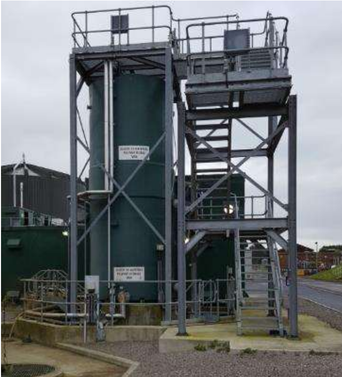
Photo 9: Polyelectrolyte mixing and storage tank
