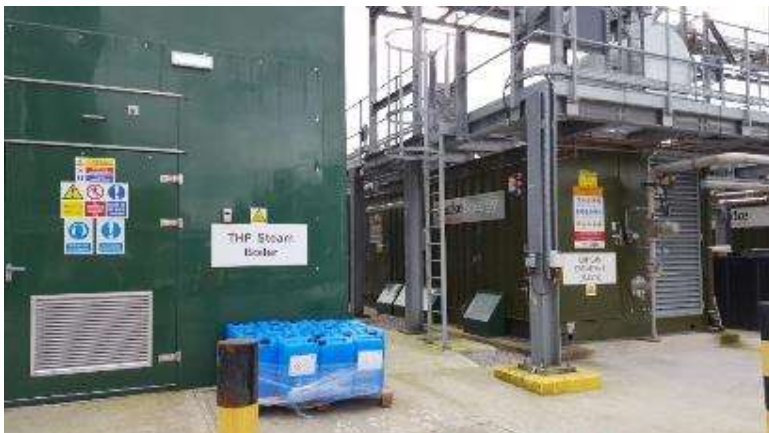
Photo 12: THP boiler and CHP engine
