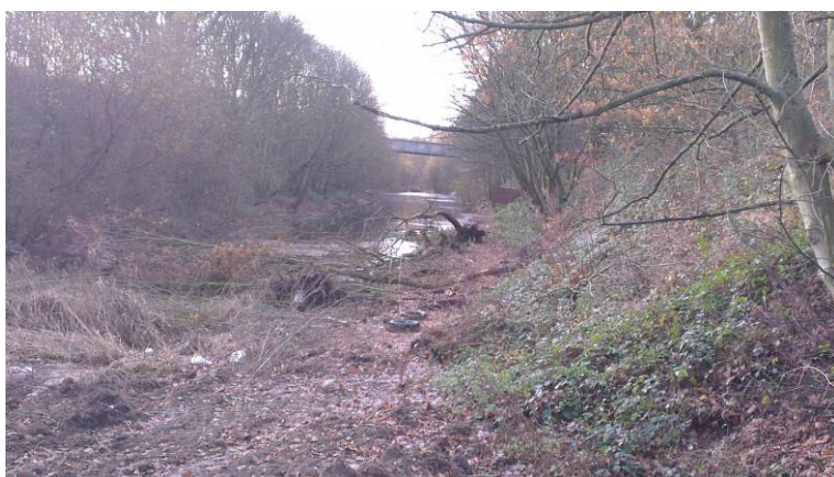
View looking south along flooded section of railway cutting towards road bridge and with views of elf seeded scrub and examples of fly tipping
