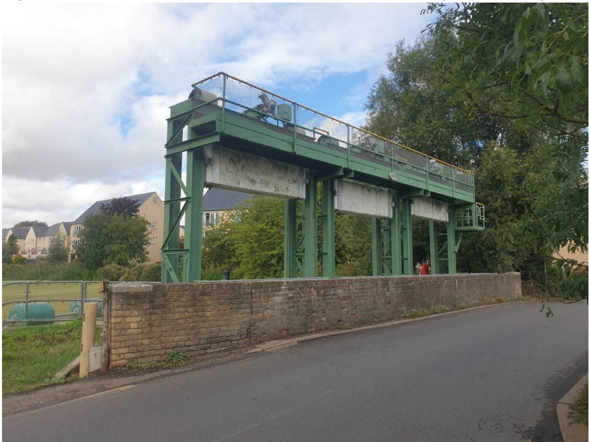
Figure 6: EA sluices – view upstream from road, at south bank of road bridge
