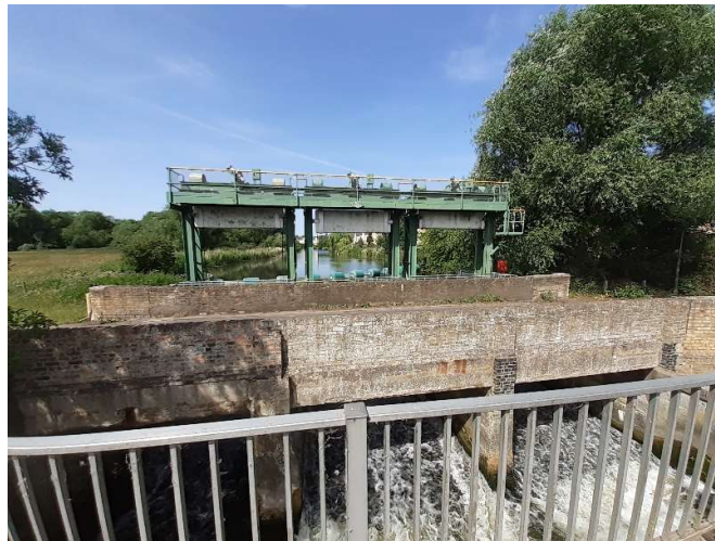
The River Great Ouse and its structures
