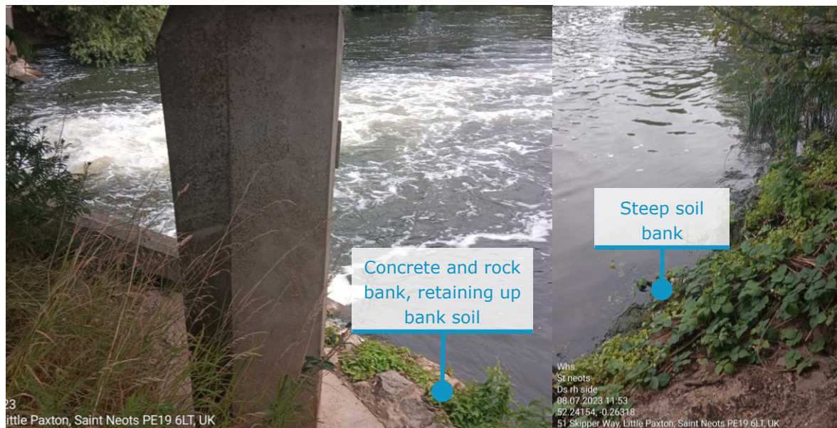
Figure 12 Outfall location, left showing bank material near wingwalls, right showing natural bank material (soils) further out from wingwalls
