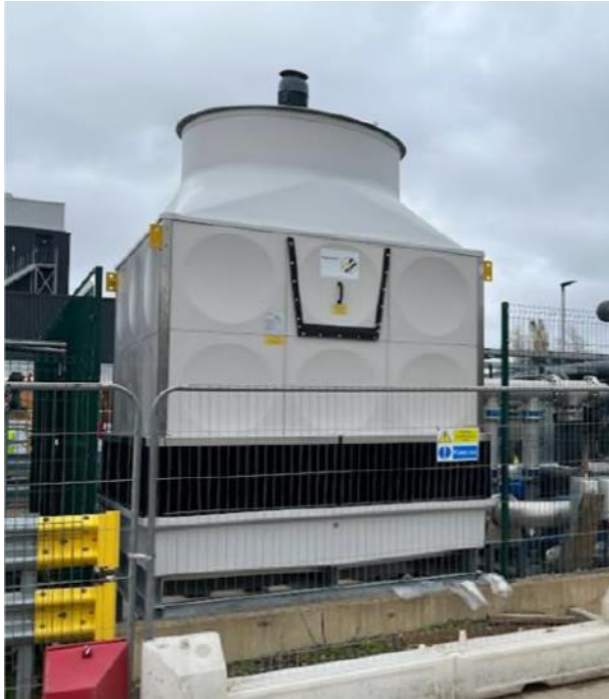
Figure 3-3 - Kelvion Polacel cooling tower photograph
