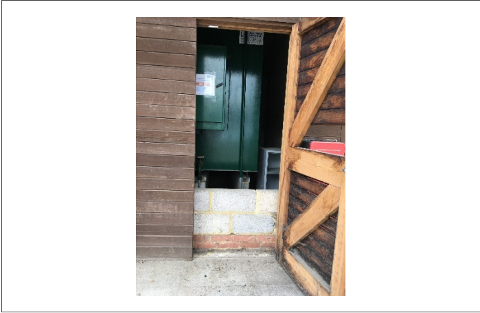
07: Vodafone (Fuel Storage Tank)
