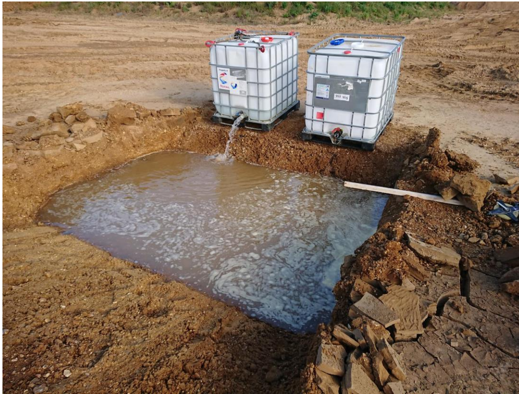
Photograph No. 1: Trial Pit 1 (2 nd May 2019) - filling trial pit with water. Pit dug by loading shovel.
