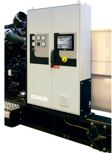
Embedded cabinet APM802 on genset.
