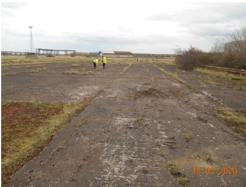
Plate 24 – View looking east southeast showing a hardstanding area. It was noted that the hardstanding surface is ‘wavy’ and cracked, again providing
