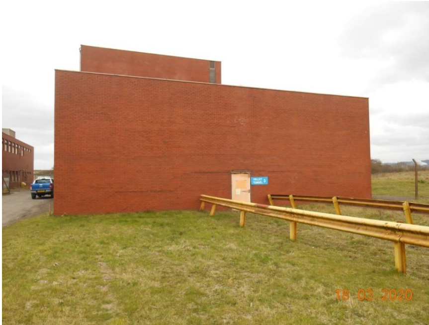
Plate 20 – View looking west showing deformation across the Pellet Tunnel building. It is noted that the extent and direction of the tunnels are not known at the time of this report issue, however STSC have indicated that these records should be available for release. The barriers leading to the structure again delineate the corridor of buried underground services and high voltage cables.
