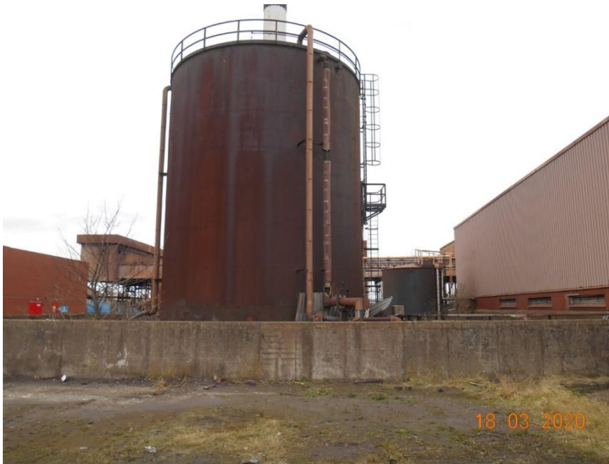
Plate 27 – View looking west northwest showing diesel tank and surrounding concrete bund wall.
