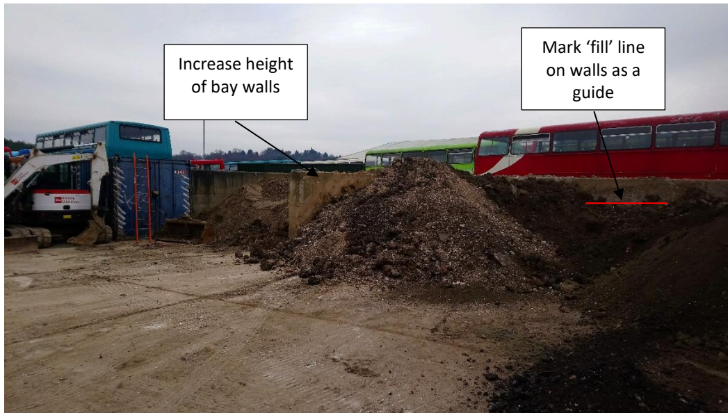
FIGURE 4.2: PHOTOGRAPH SHOWING OVERFILLED BAYS
