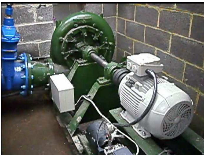
Figure 16 : Francis installation at Ladygrove Mill
