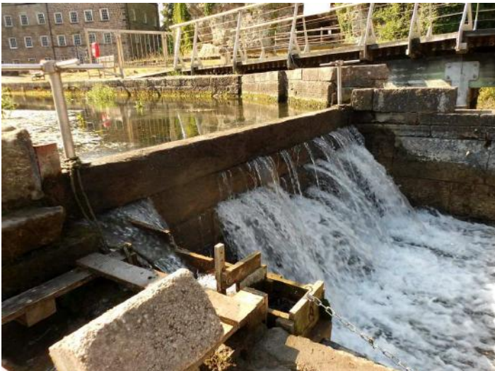
Figure 7 : Leakage flow through the wheelpit stop-logs (7/9/21)
