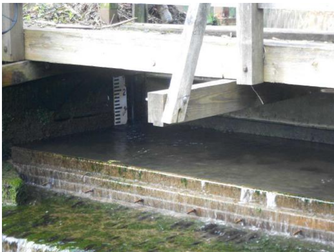
Figure 9 : New upstand with water level gauge
