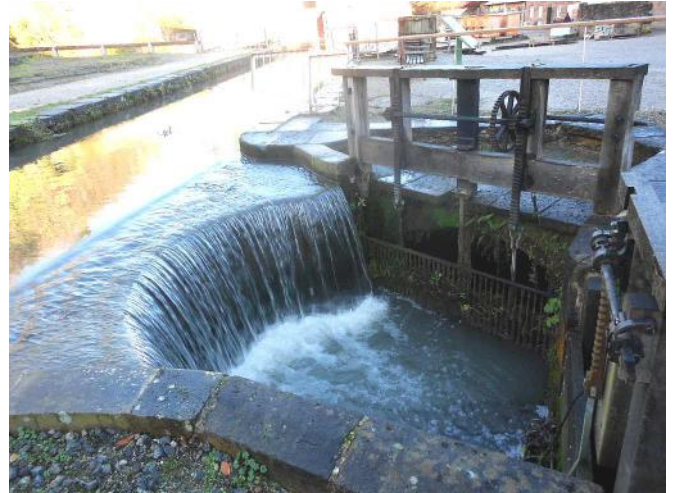
Figure 4 : Discharge into the Canal from the Horseshoe Weir on 26/11/21
