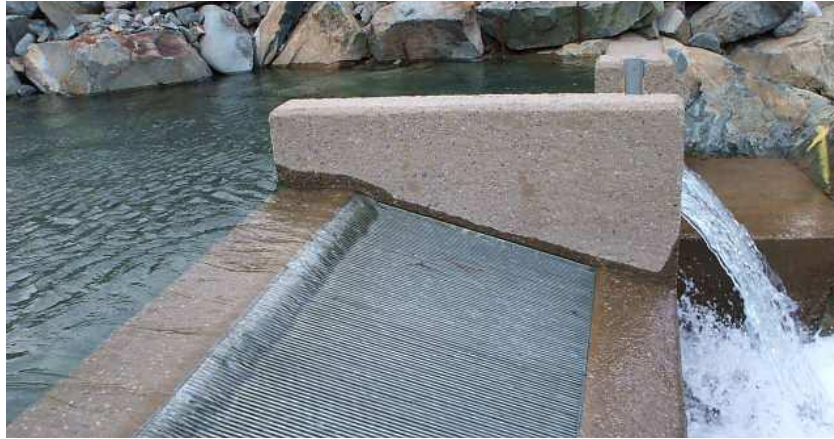
Figure 18 : Overflow bar screen (Tyrolean)
