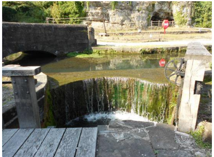
Figure 8 : Horseshoe Weir – deprived by leakage flow (7/9/21)
