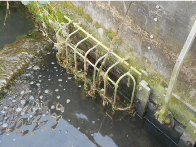
Figure 28 : Rectangular orifice limiting flow from the Horseshoe Weir into the Canal
