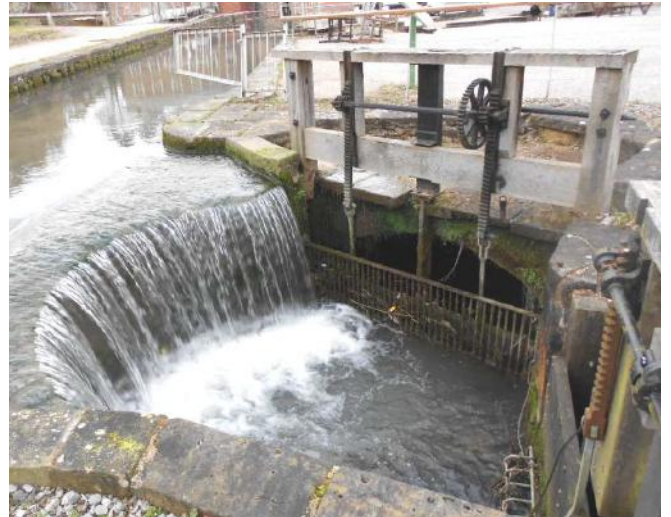
Figure 29 : Side culvert & sluices taking excess flow from the Horseshoe Weir back to the Derwent
