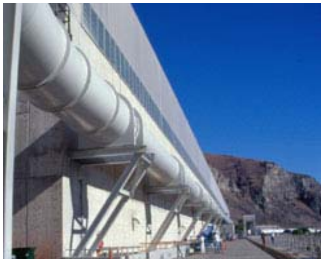
Plate 3.15 The bypass pipe traversing the dam (Chelan County PUD).
