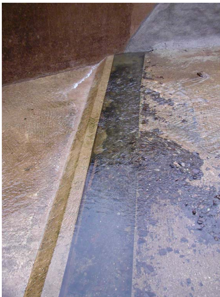
Plate 3.15 Eel bypass trough at Backbarrow hydropower scheme, R. Leven, Cumbria (Spiby, 2004).
