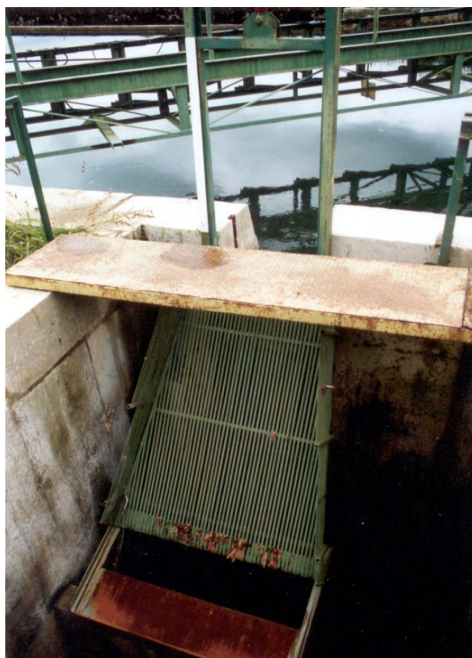
Plate 7.3 A Wolf trap photographed at Halsou, France. Water is strained through a set of parallel rods or slats that run along the length of the channel. These are spaced at about 6mm apart, allowing water to pass through, while fish are flushed along the slats and into a holding tank at the downstream end.
