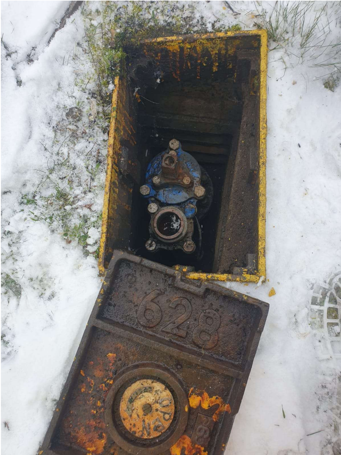
Annex G – Photograph of Fire Hydrant
