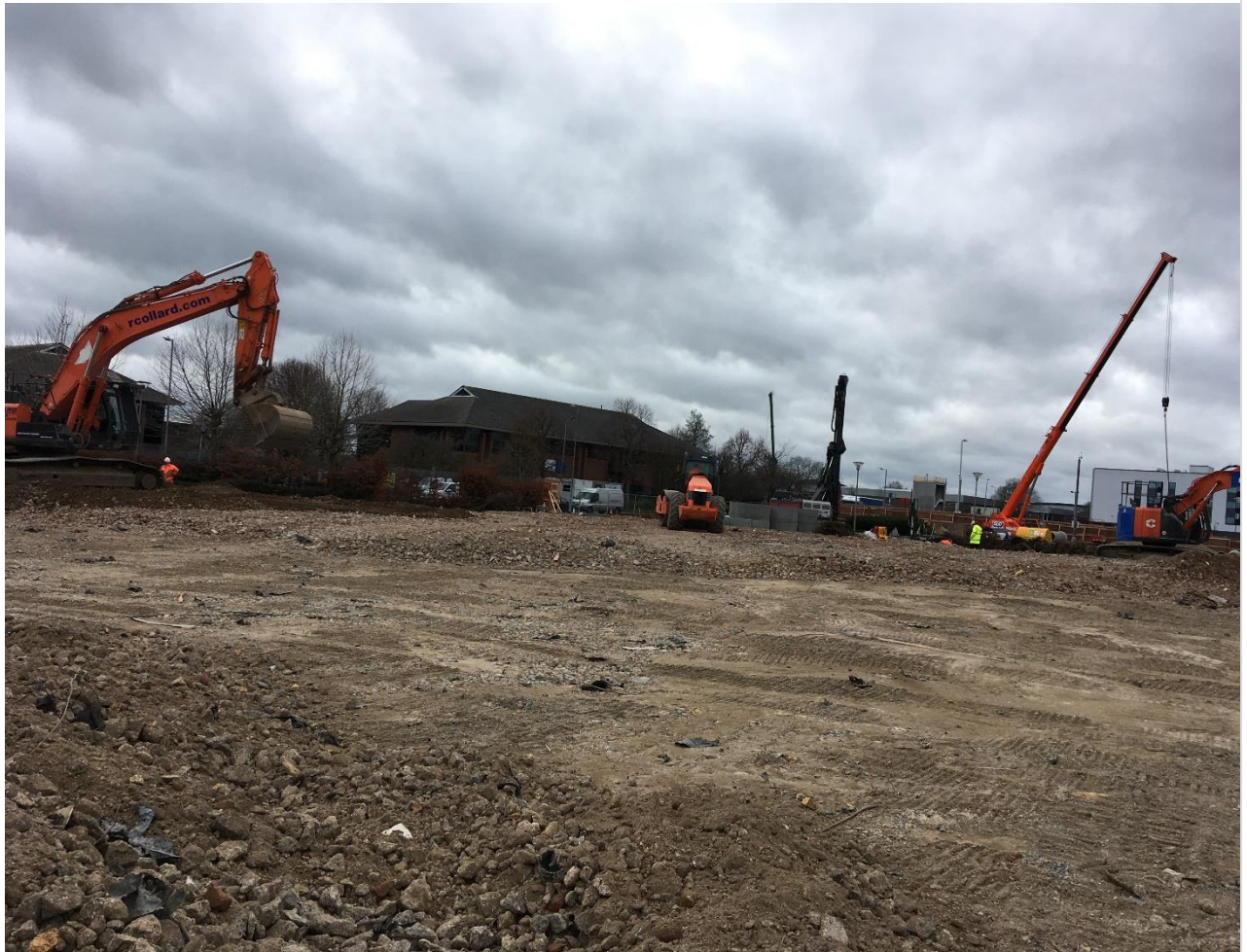
Photograph 2 – central area to be levelled and proof rolled, with Thames Water sewer diversion and sheet piling in south west corner.
