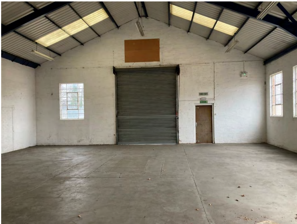
Photograph 4 – Typical internal warehouses at the Site with manual roller shutters (658 Ajax Avenue)
