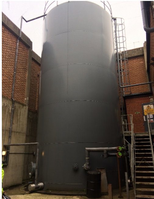
Photo 1. Bulk fuel storage tank, Building 7
