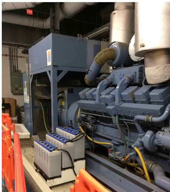
Photo 10. Building 5, ground floor generator with separate (elevated) day tank and brick bunding
