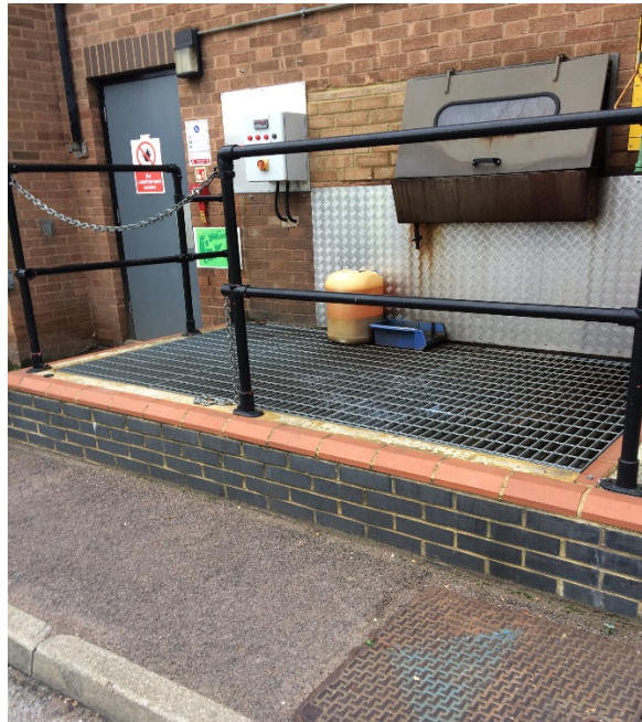
Photo 5. Bulk tank offset refilling point with containment
