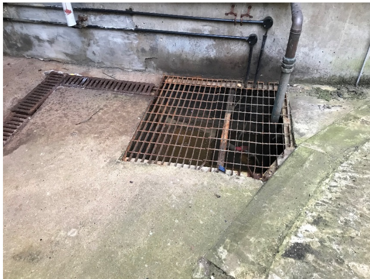
Photo 4. Sump for draining containment bund to bulk fuel storage tank
