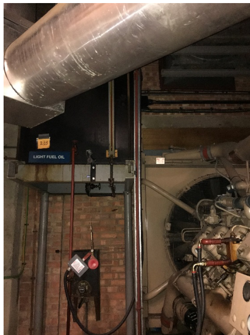
Photo 14. Building 27 Day tank (at elevation) and adjacent generator (right of frame)
