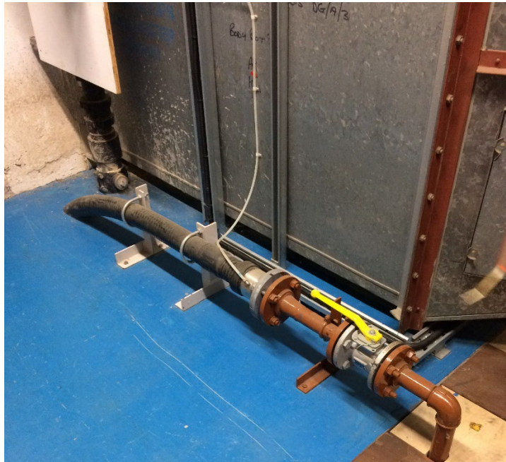
Photo 11. Ingress of fuel distribution pipeline connecting generator in Building 5 to main bulk fuel tank (and pump sets) in Building 7
