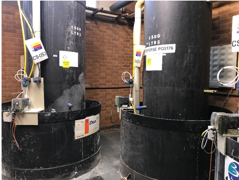
Photo 7. Boiler treatment chemical storage, internal to Building 7
