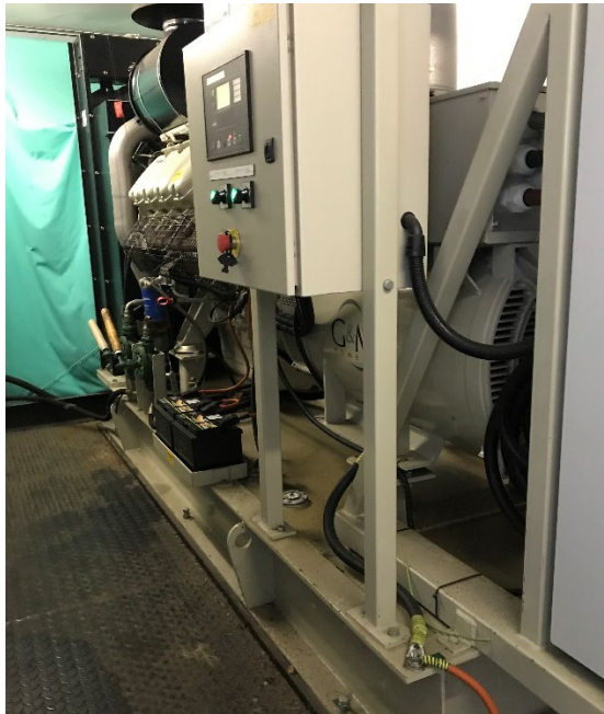
Photo 9. Building 9, generator with integral day tank
