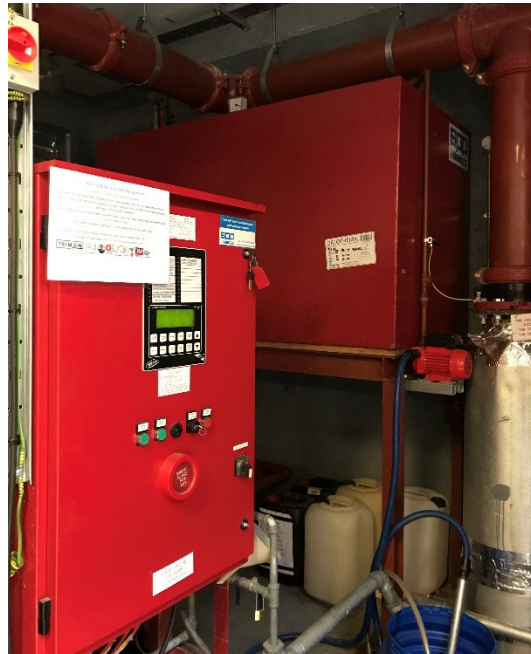
Photo 13. Fire water pump house day tank
