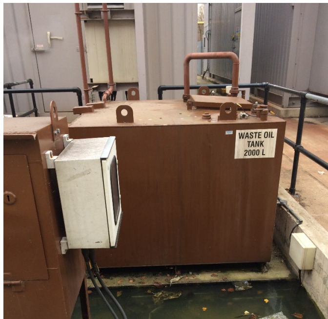
Photo 12. Waste Lubrication Oil storage tank adjacent to CHP
