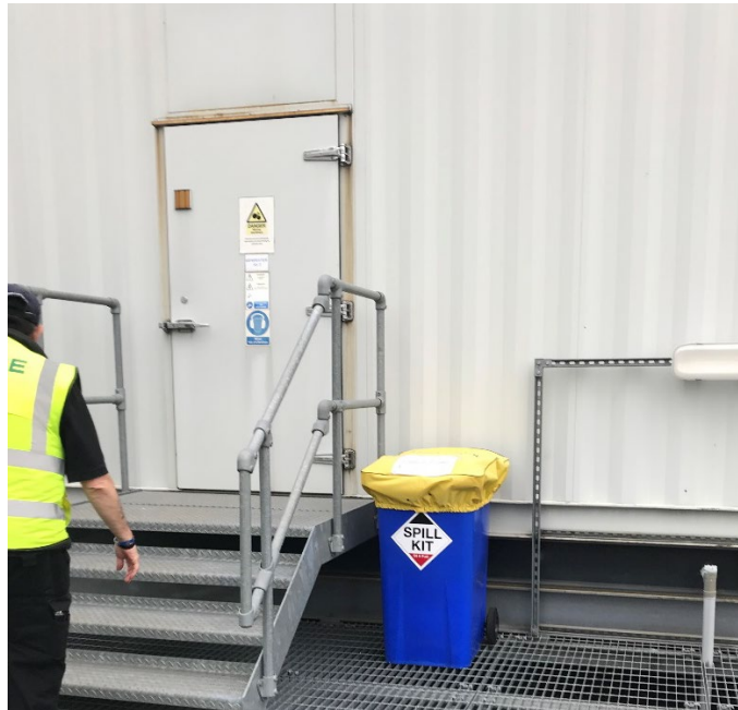
Photo 8. Building 9, roof top generator container with spill kit
