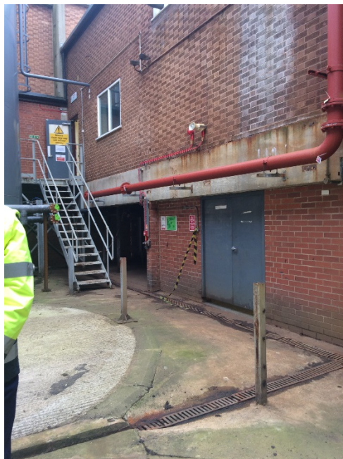
Photo 2. Containment and drainage for bulk fuel tank, Building 7
