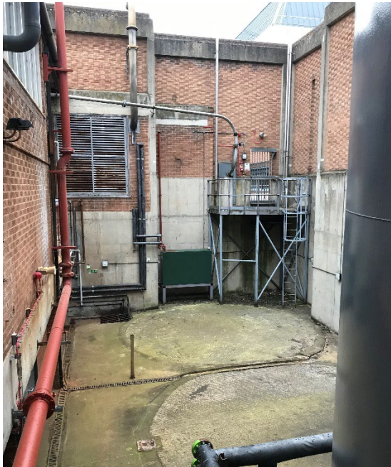
Photo 3. Containment and drainage for bulk fuel tank, Building 7. Day tank for generator in rear of view
