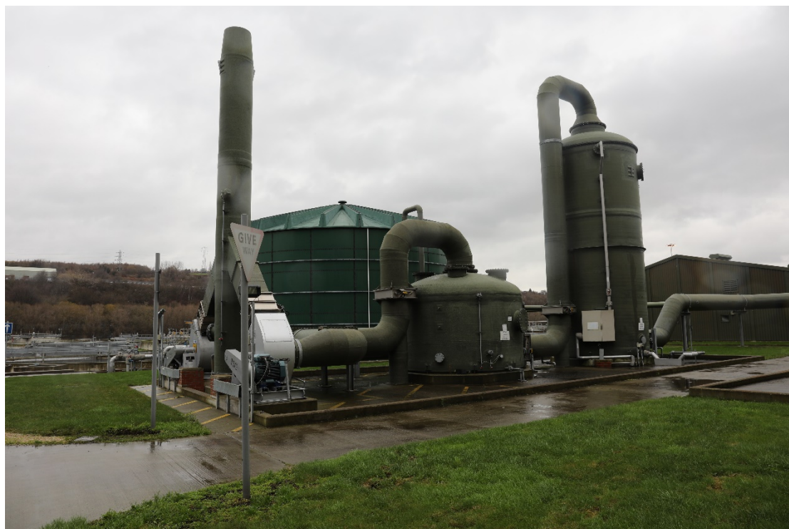
Figure G Odour control unit
