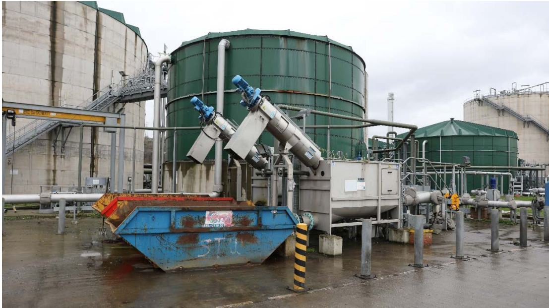
Figure E Enclosed rotating sludge screens
