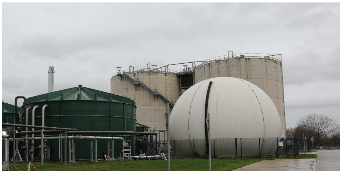
Figure I Biogas holder (with digesters behind)
