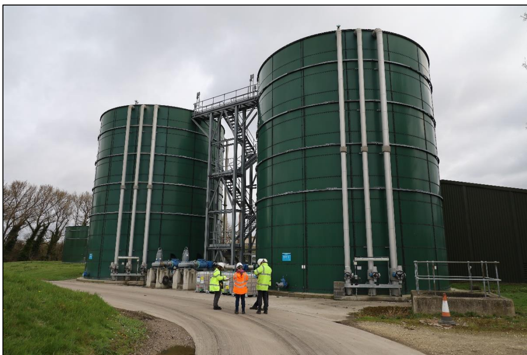
Figure 9. Thickener feed tanks
