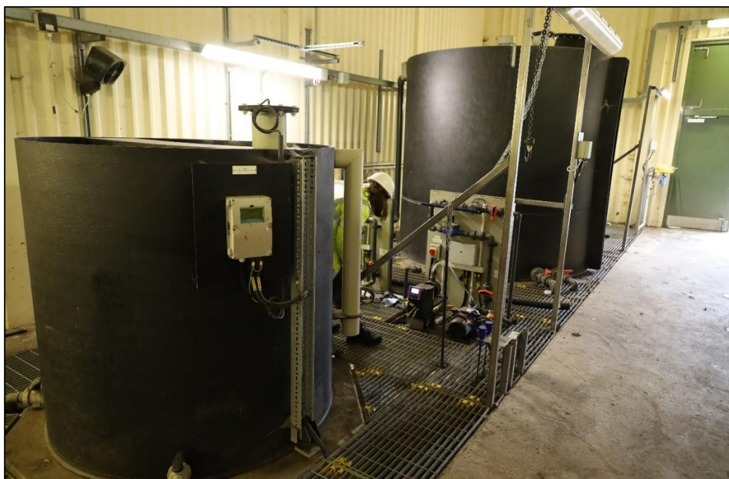
Figure 11. Polymer tanks in drum thickener building.
