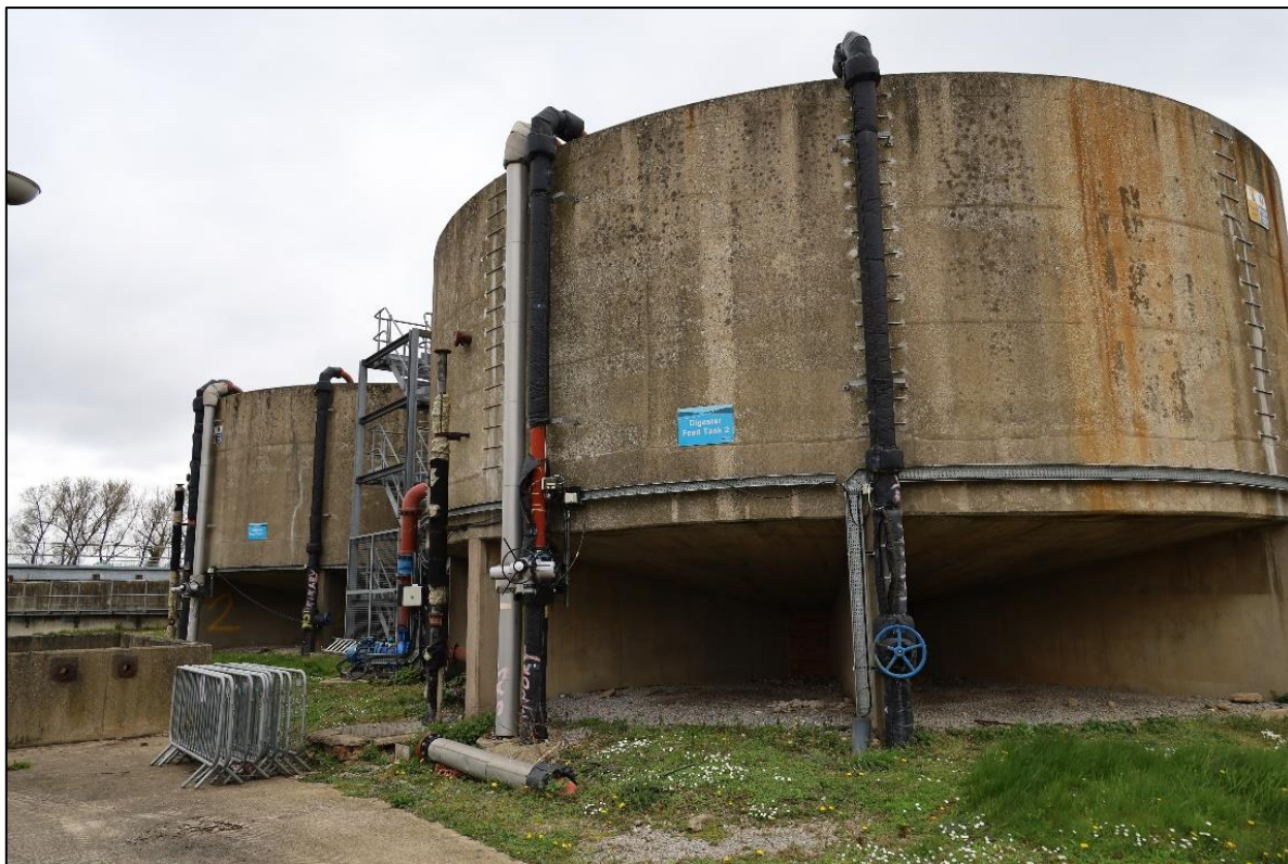
Figure 12. Digester feed tanks (2.no)
