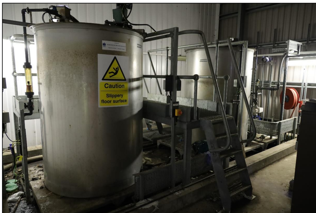
Figure 15. Polymer tanks within centrifuge building.
