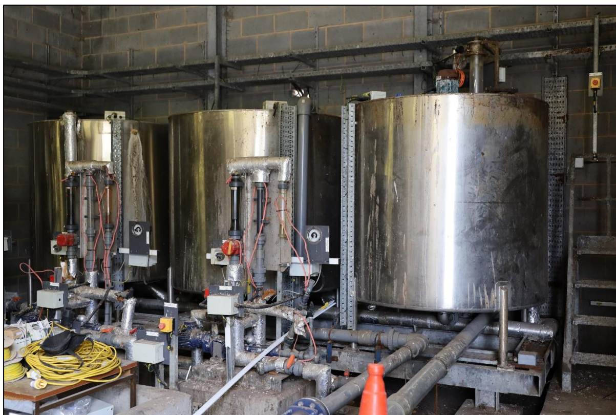
Figure 10. Polymer tanks in GBT building.
