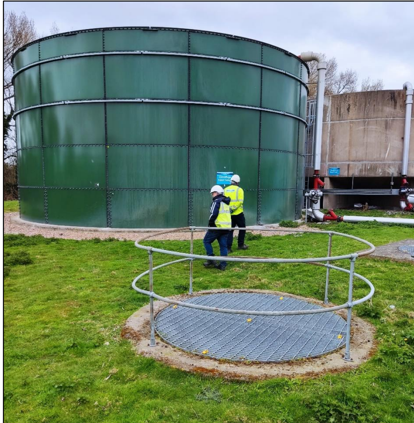
Figure 26. Outlet open well near steel centrifuge feed tank.
