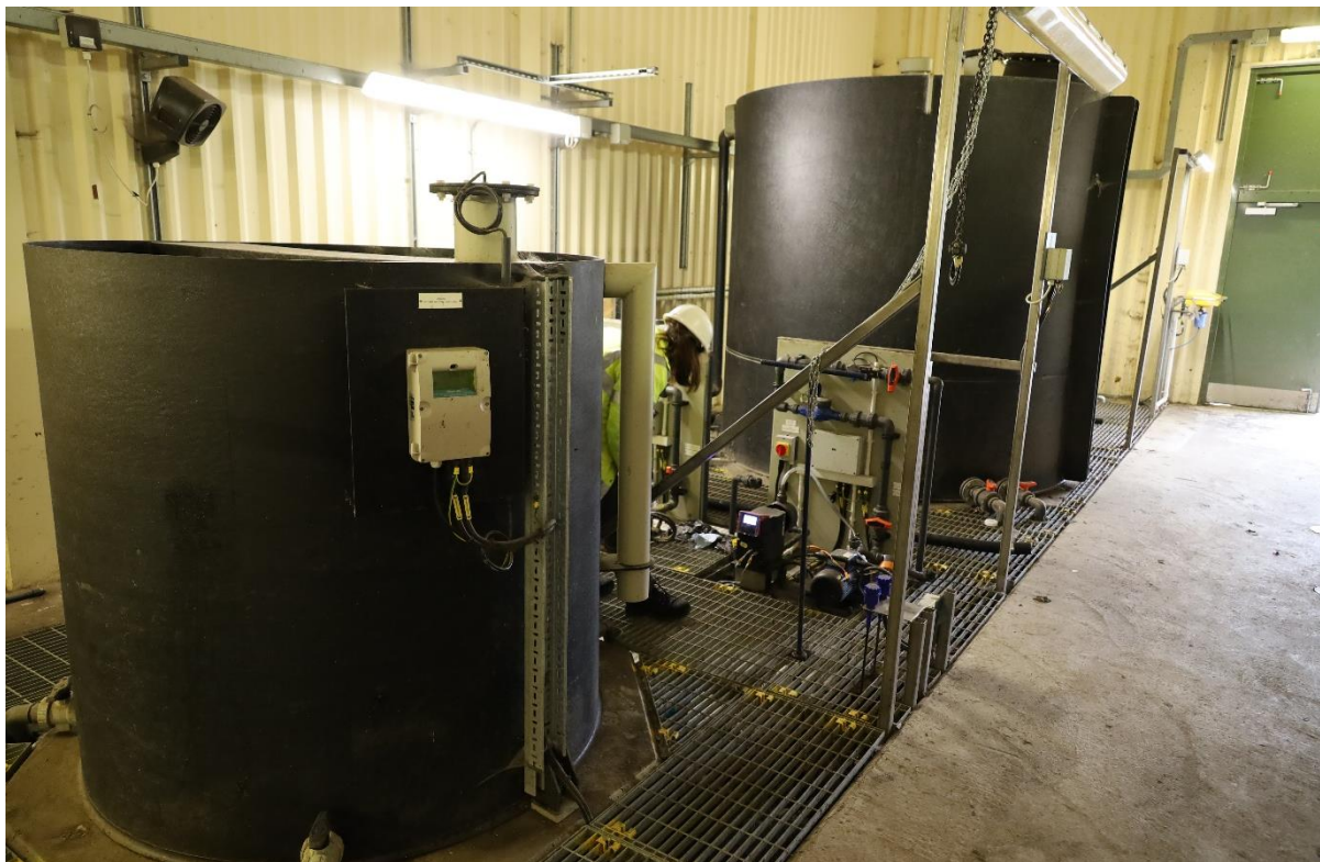
Figure F Polymer tanks in drum thickener building
