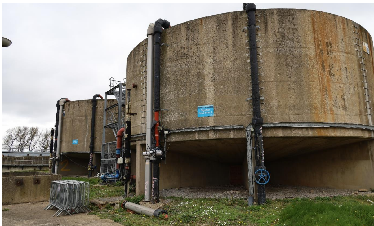
Figure G Digester feed tanks
