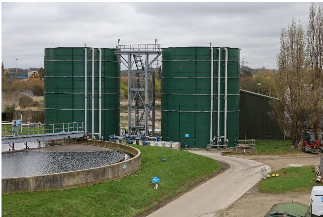
Figure D Thickener feed tanks
