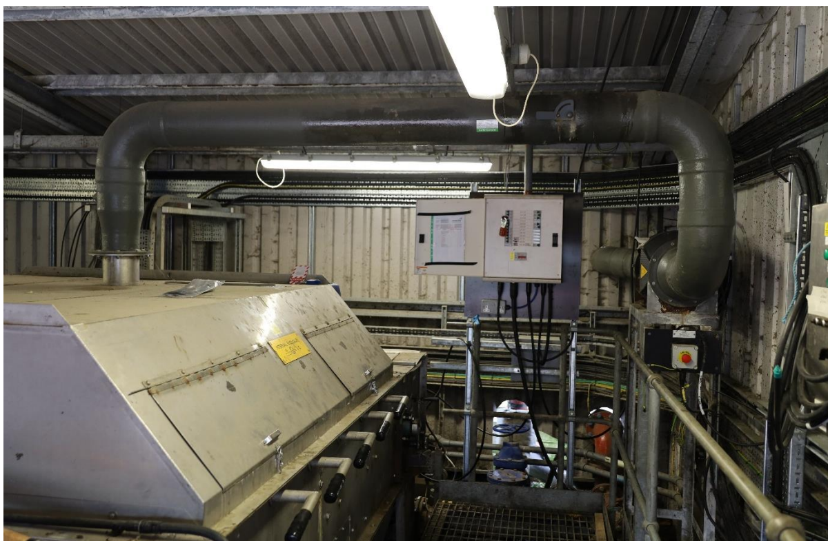
Figure E Air extraction from GBT
