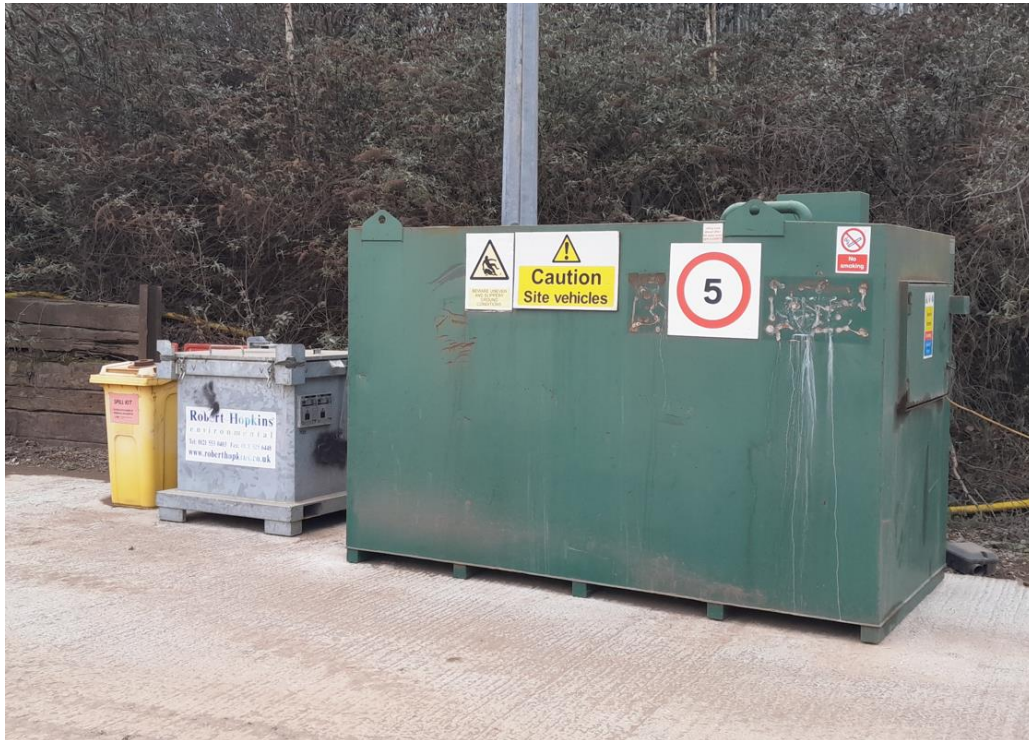
Photograph 6-6: Diesel storage AST
