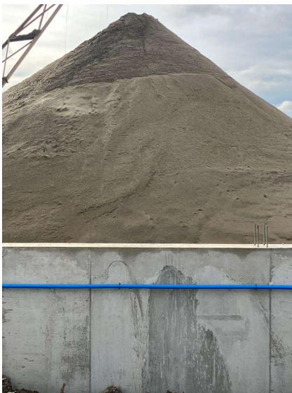
Photograph B – View showing stockpile of material on Hanson site, clearly exceeding height of RMS boundary wall.
