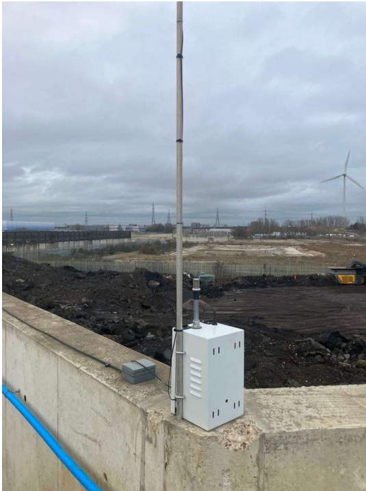
Photograph A – View showing northern boundary wall of RMS site and dust monitor. Hanson store and crush plantings on the other side of the wall. A compact crusher is visible in the photograph.
