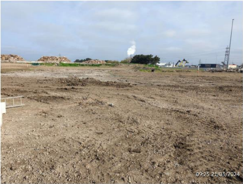
Photographs 12, 13 and 14 showing the current status of storage area after the decommissioning works have been completed
