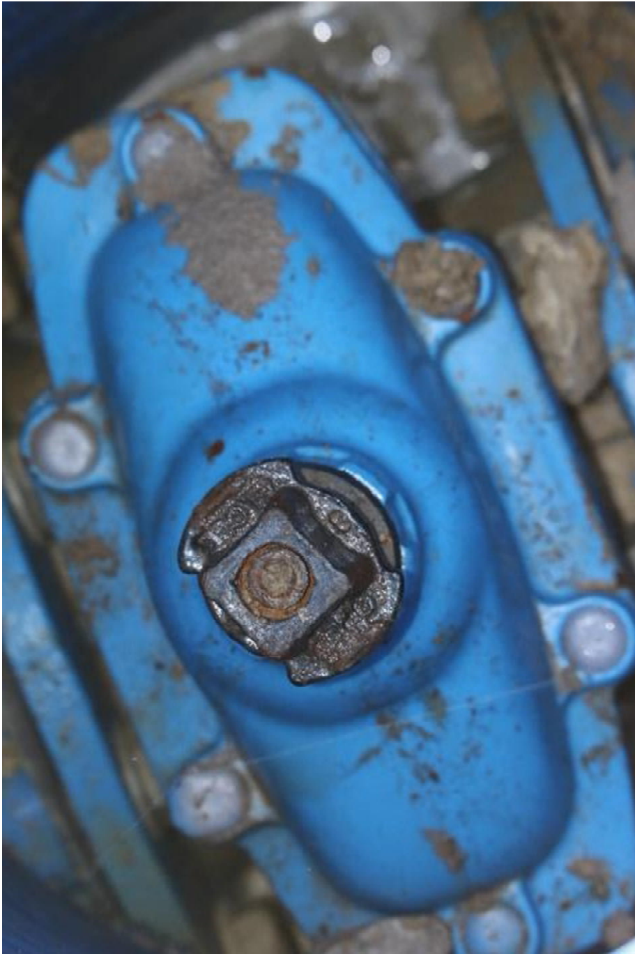
Picture 9 Closed valve with handle removed coming out of Separator
