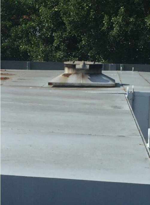
Figure 9: Unit 2 generator exhaust
