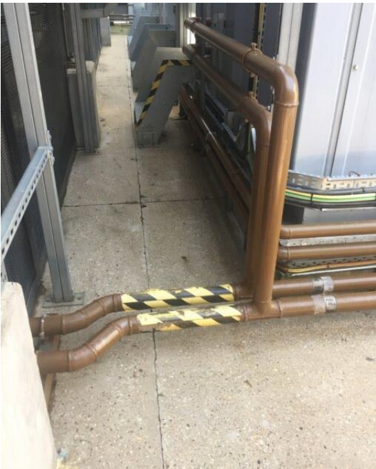
Figure 10: Unit 2 fuel pipework
