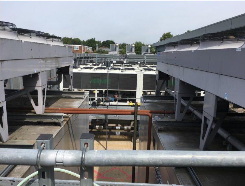
Figure 11: Unit 3 view of S120/S130 generator exhausts
