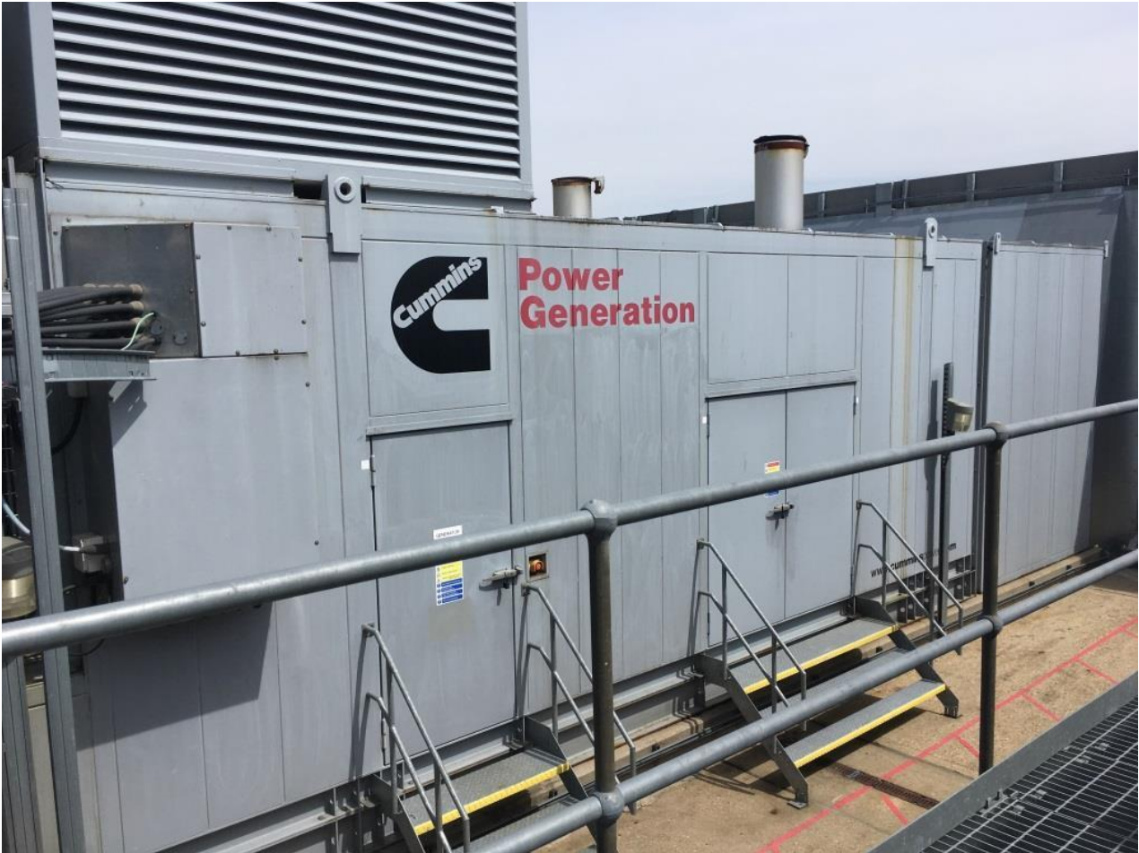
Figure 1: Redhill data centre diesel standby generator
