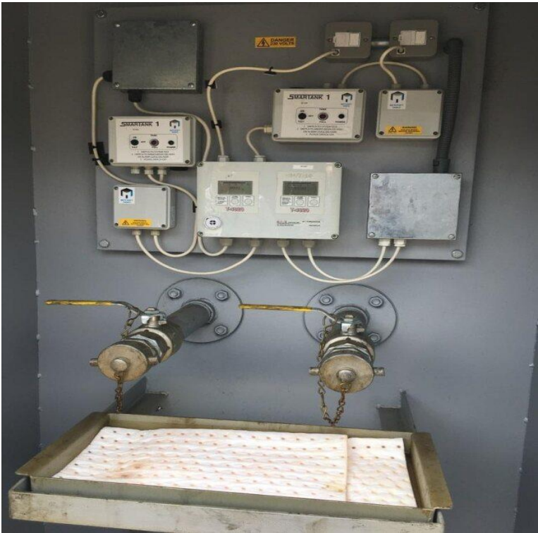
Figure 5: Unit 3 bulk tank fill points and alarms within fill point cabinet
