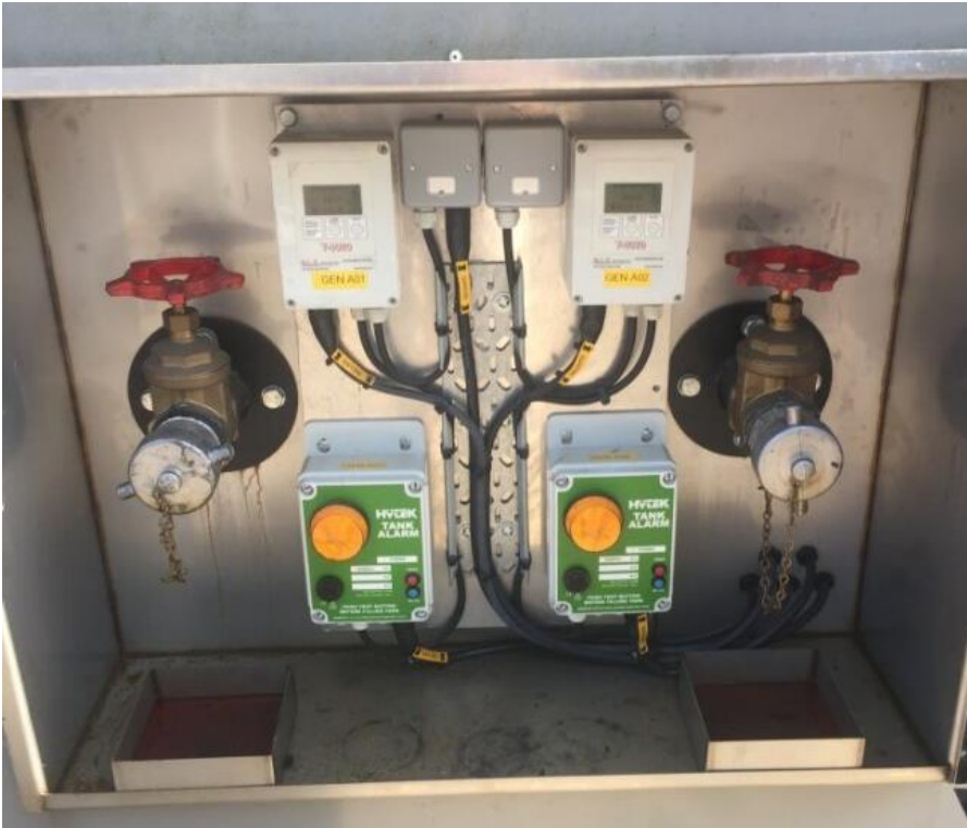
Figure 4: Unit 2 aboveground tank fill points and alarms within fill point cabinet
