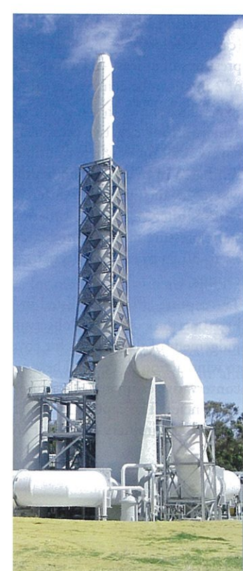
Scrubbers and Stack at Wastewater Treatment Plant.
