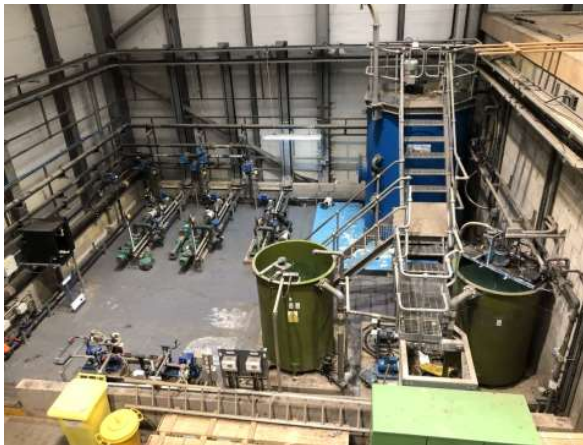
Photo 14 – Polyelectrolyte preparation area
