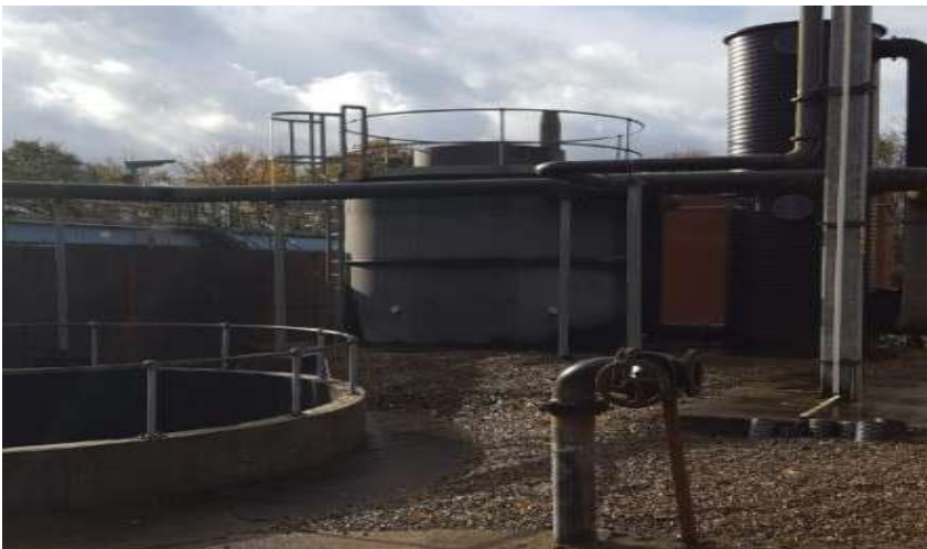
Photo 5 – OCU connected to the unthickened sludge tank
