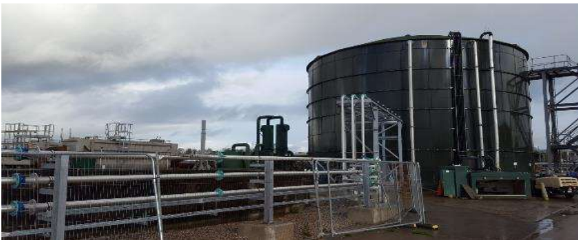
Photo 7 - EEH feed tank and OCU
