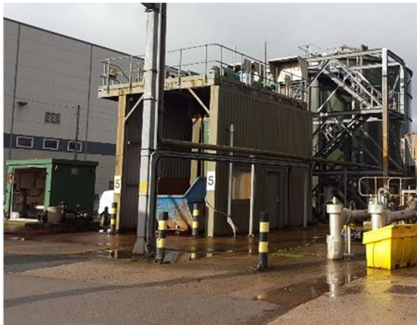
Photo 3 – Screening unit and screenings skip
