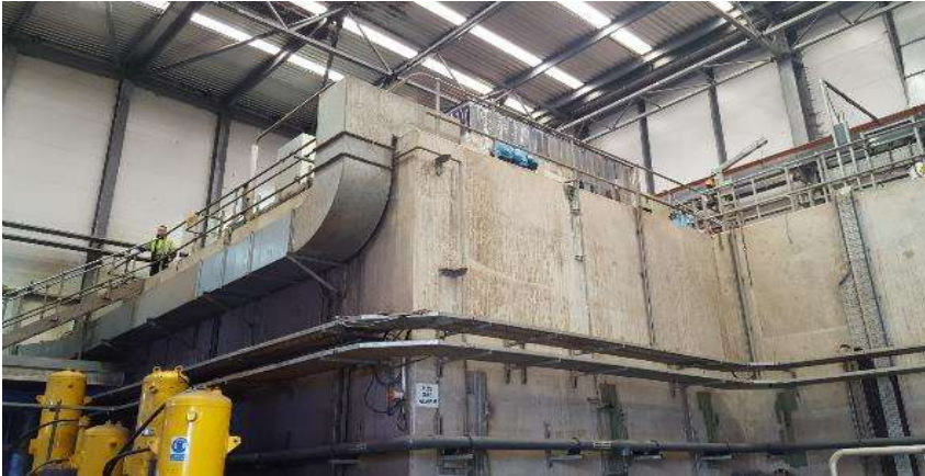
Photo 6 – GBTs within the building
