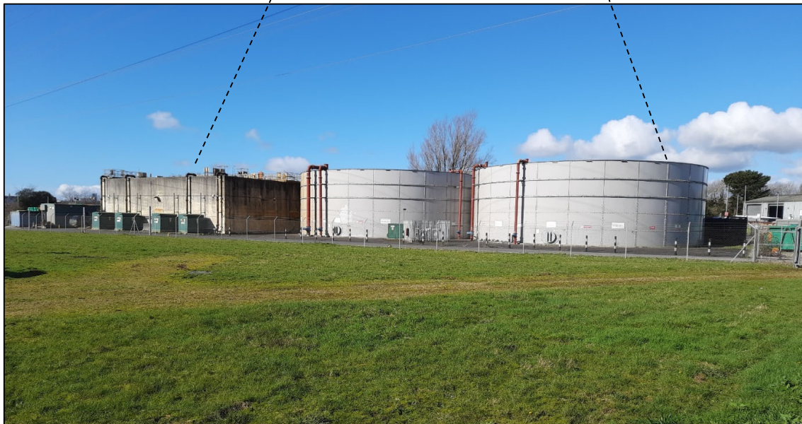
Plate 1: Leachate Treatment Plant, looking southwest from the lagoon pumping station, Chelson Meadow, Plymouth 2021. Infrastructure components from left to right are: Sequential Batch Reactors (SBRs), STOR 2 & STOR 1
