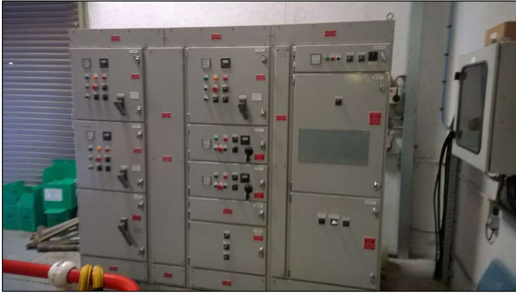
Plate 3.3.4: Control panels (MCC) that operate the three pumps, within the PLS
