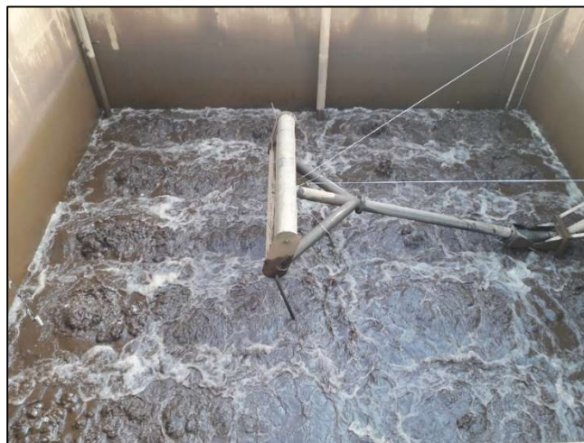
Plate 5.9: Blowers in 'Hand' mode aerating the source liquor prior to transfer to the receptor SBR
