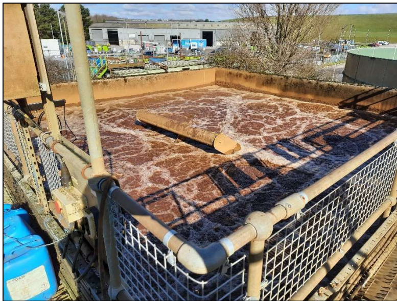
Plate 5.5: Blowers aerating liquor in the SBR during the Mix/React phase, 2021
