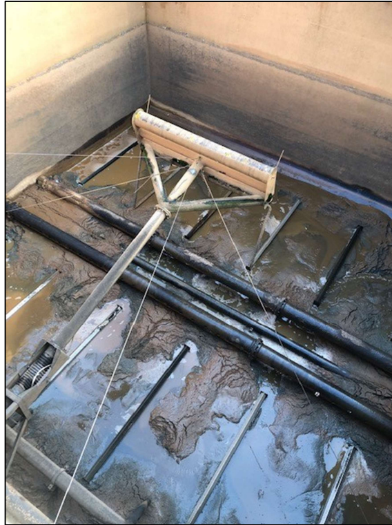
Plate 5.16: Empty SBR requiring cleaning, showing residual sludge in the bottom
