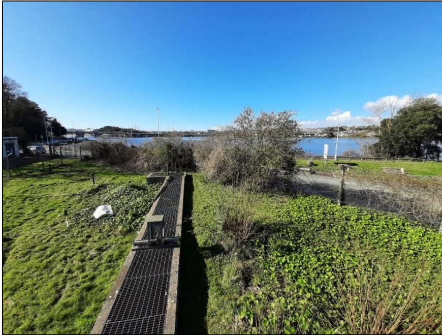
Plate 3.7.1: Discharge channel at the point where it meets The Ride and travels below ground
