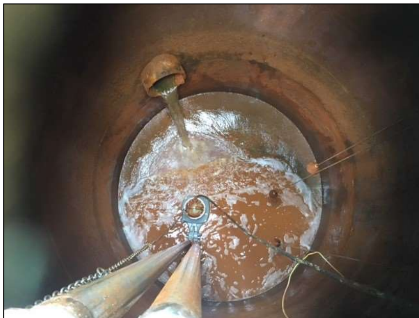
Plate 2.10: Looking into the North Leat leachate well, showing the pump and floats, October 2018
