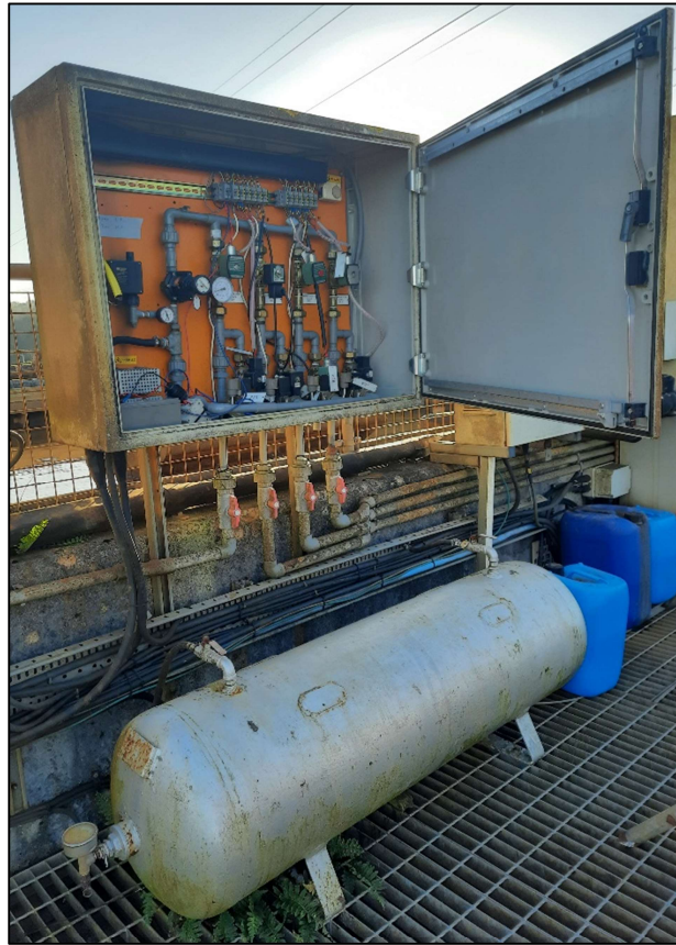
Plate 3.4.8: Receiving vessel for compressed air, showing control cabinet above for regulating each SBR Decant Arm
