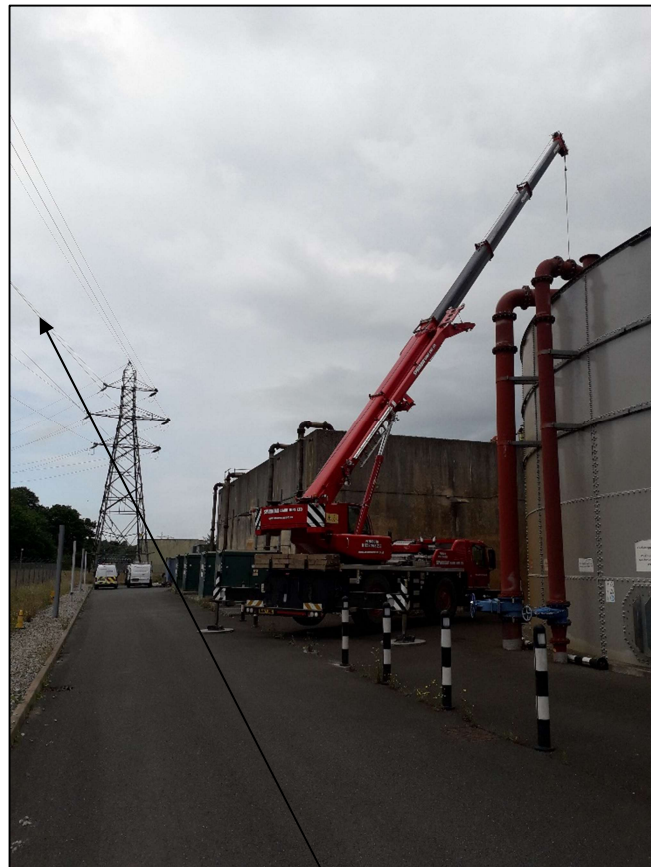
Plate 4.1.2: Crane position for lifting pumps in SBRs 2 & 3, showing overhead power cables on the left
