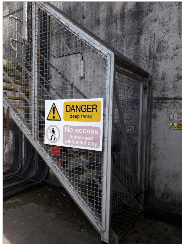
Plate 9: Access gate to SBRs, which must be relocked after sampling is completed or when absent from the LTP temporarily
