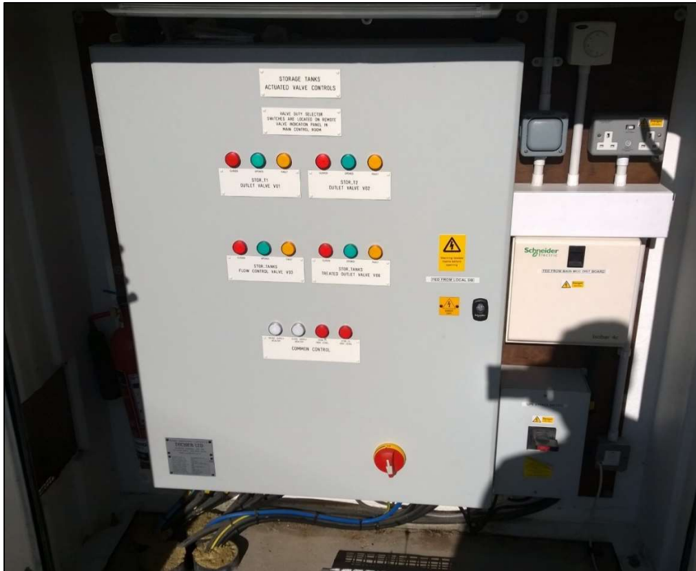
Plate 3.2.5: Control cabinet for the STOR valves, housing electric panels & the UPS
