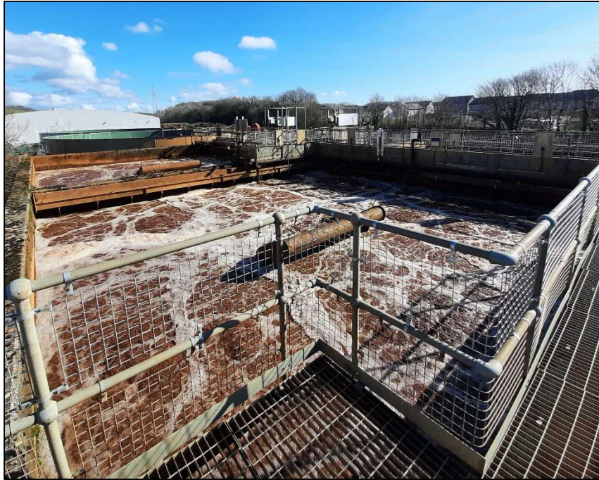
Plate 3.4.13: Liquor within SBR being aerated when blowers and diffusers are operational
