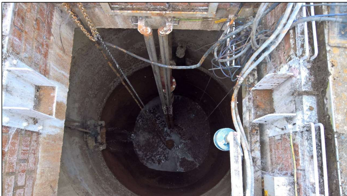
Plate 2.16: Looking into the South Leat leachate well, showing the pump in the bottom of the well, April 2019
