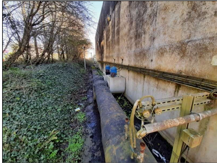
Plate 3.4.5: Northern edge of the SBRs showing leachate inlet pipe from the PLS and associated valves
