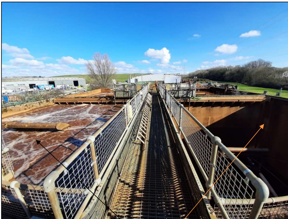
Plate 2.7: Top of the treatment tanks SBR1 & SBR4 viewed from the access walkway, showing aeration during the treatment process in SBR1 left of centre, 2021
