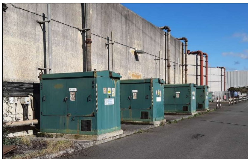
Plate 3.4.9: Blower cabinets alongside the SBR plant, 2021
