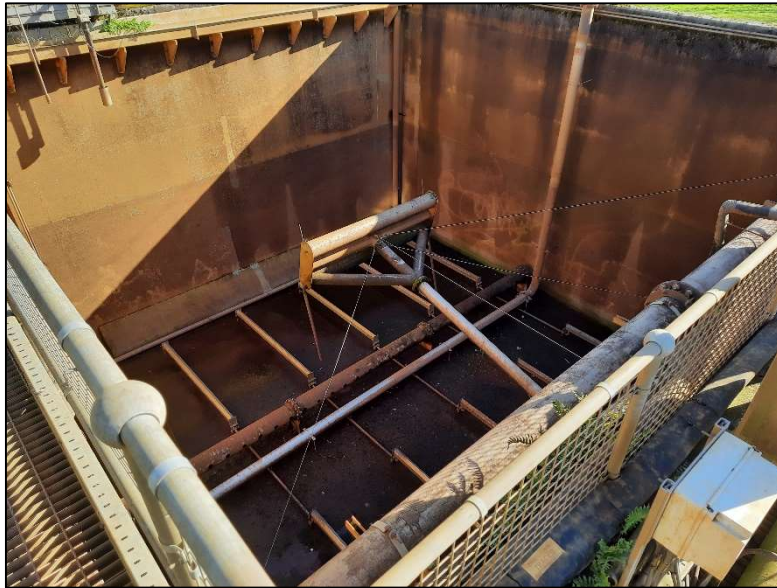
Plate 5.2: Standby SBR, left empty of sludge (bacterial biomass) and leachate, 2021
