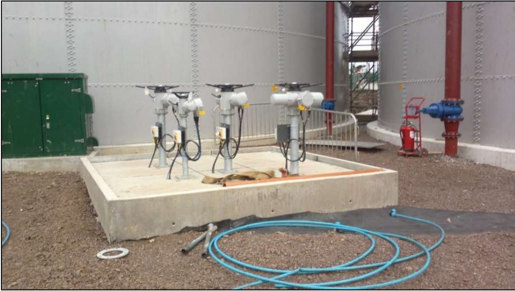
Plate 3.2.3: Completed valve chamber, minus security fence, showing control cabinet housing UPS on the left
