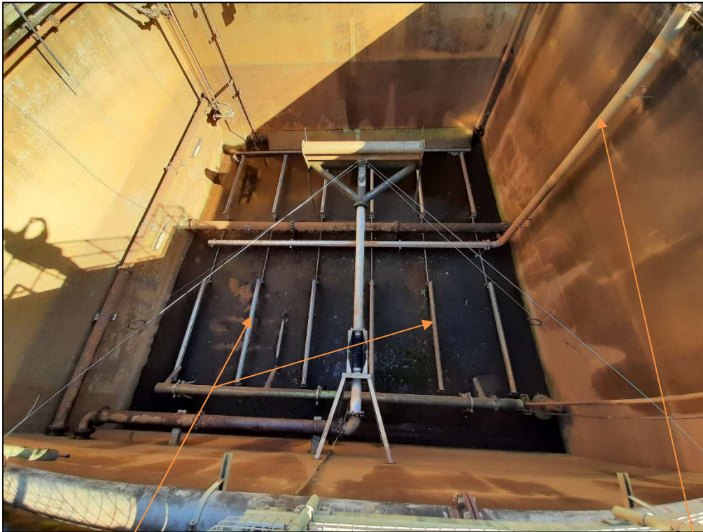
Plate 3.4.12: Diffusers (12) located at the bottom of each SBR, served by the air feed pipe
