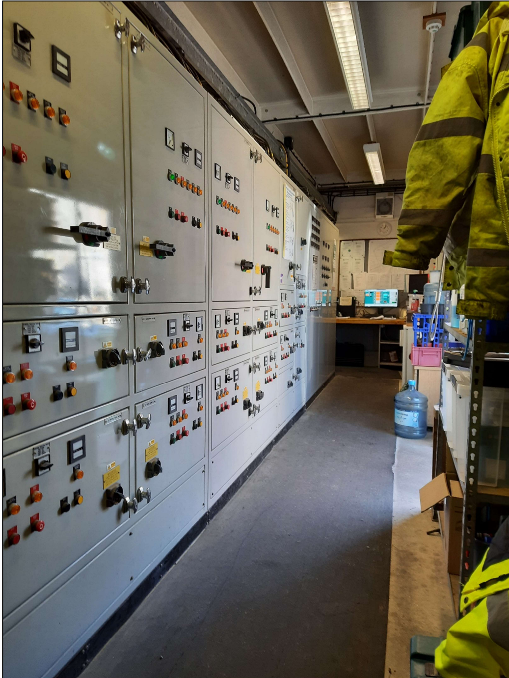
Plate 3.5.3: Control cabinets in the control room, 2021
