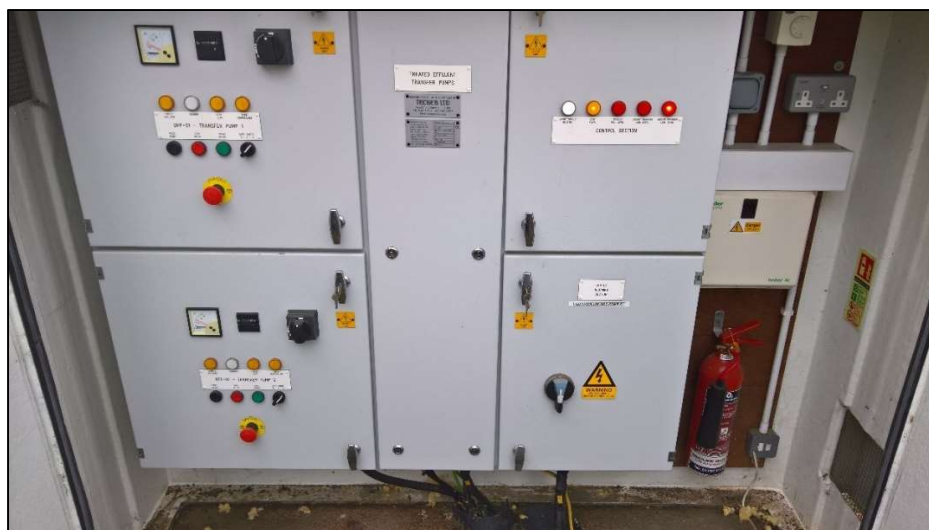
Plate 3.6.2: Control panel for the TLPS inside the cabinet adjacent to the pumps
