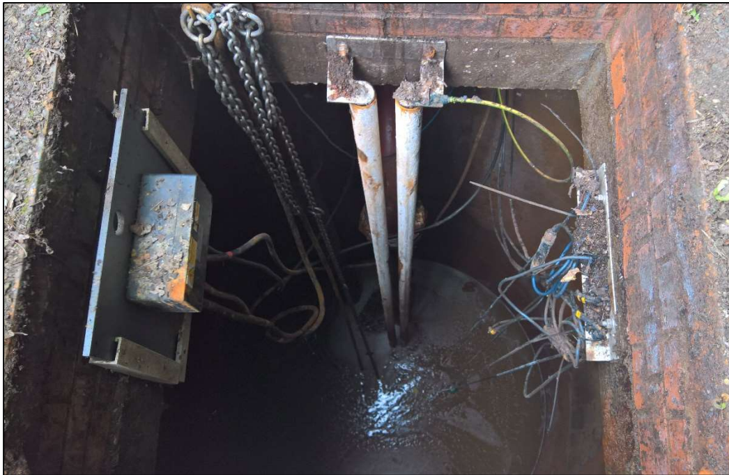
Plate 2.13: Looking into the Ride leachate well, showing the pump, floats and junction boxes, August 2018
