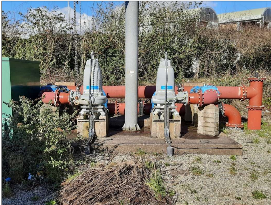
Plate 3.6.1: Treated Leachate Pumping Station showing two pumps and associated pipework
