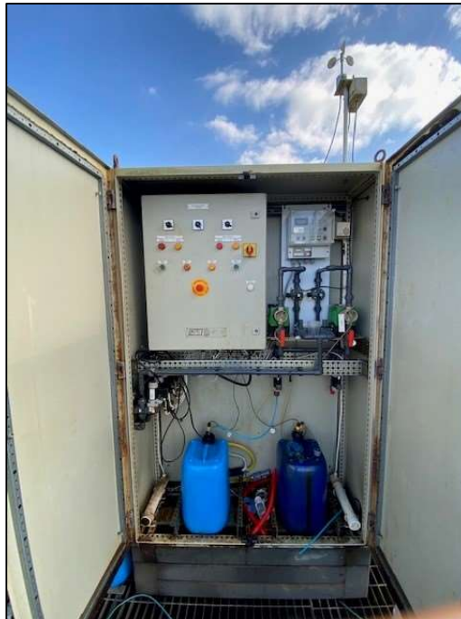
Plate 7.1: Automatic defoaming system, dedicated cabinet, LTP 2021
