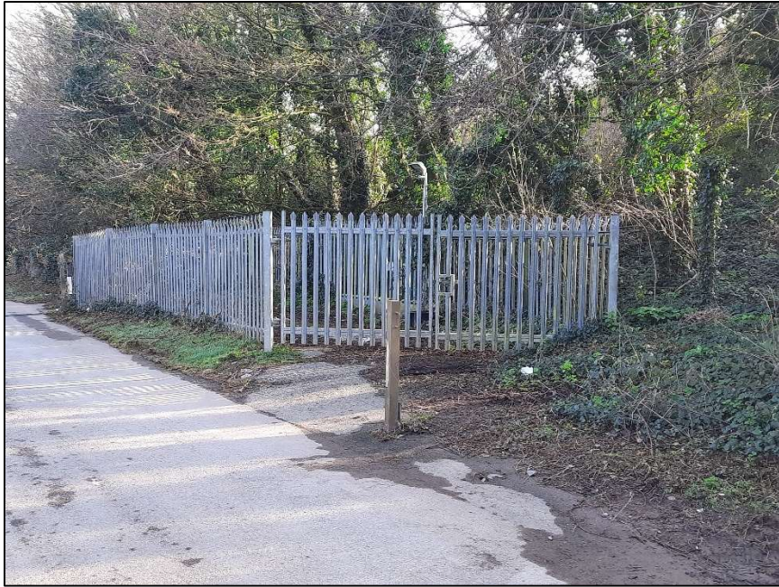
Plate 2.11: Ride Pumping Station (NGR SX50658 54756), Chelson Meadow Landfill.
