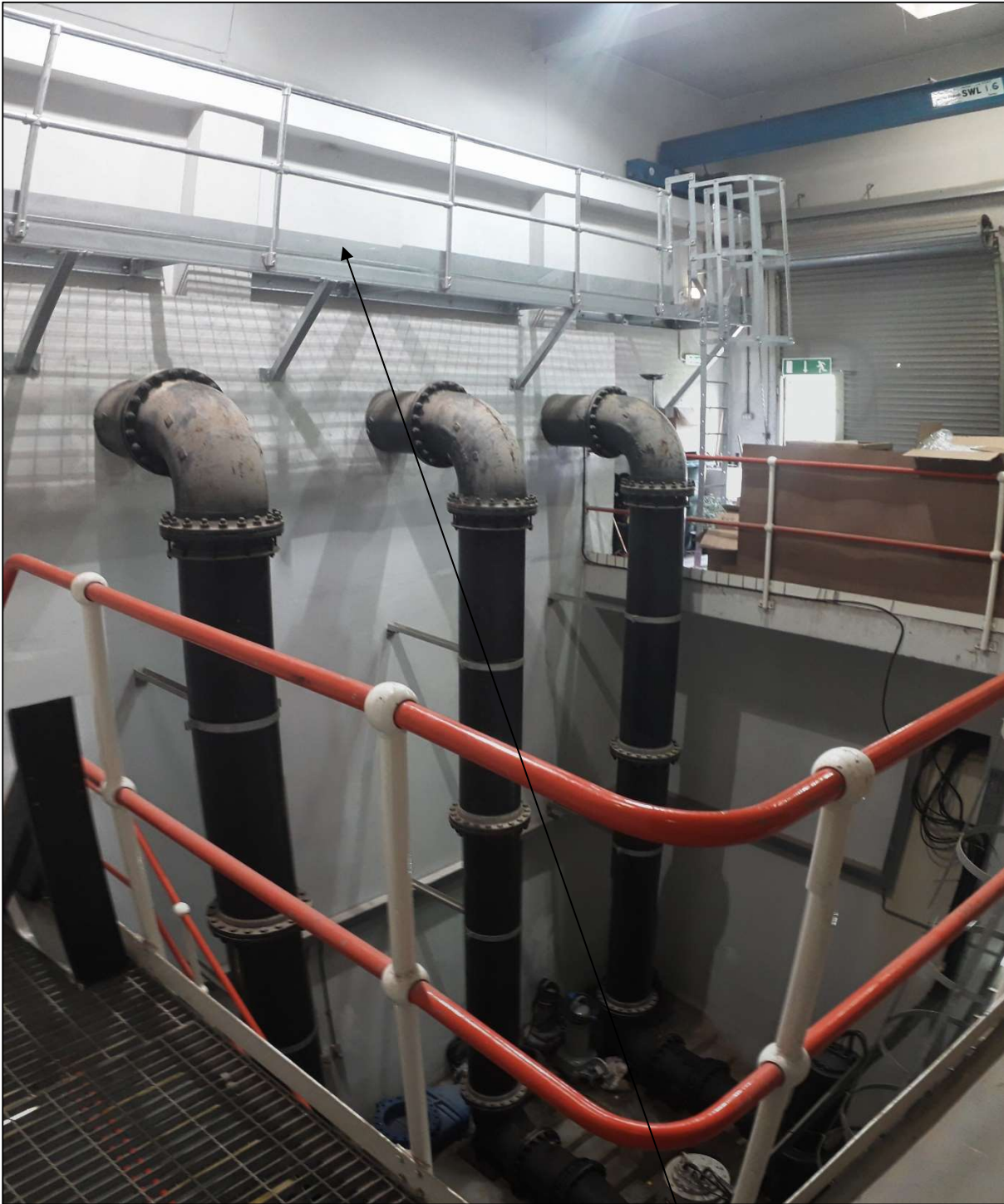
Plate 3.3.3: View of the pump outlets inside the PLS and inspection walkway used when the overhead crane is being serviced
