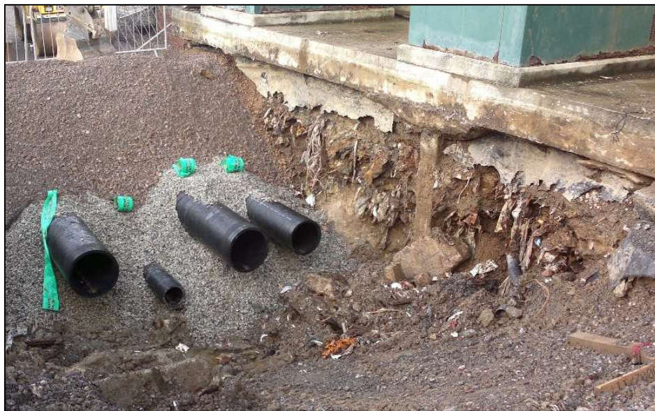
Plate 3.4.2: Excavation of historic waste mass beneath the LTP during installation of pipes serving STORs1 and 2
