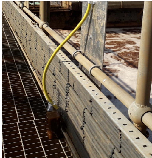
Plate 4: SBR sampling pump outlet filling a sample bottle with mixed/aerated liquor
