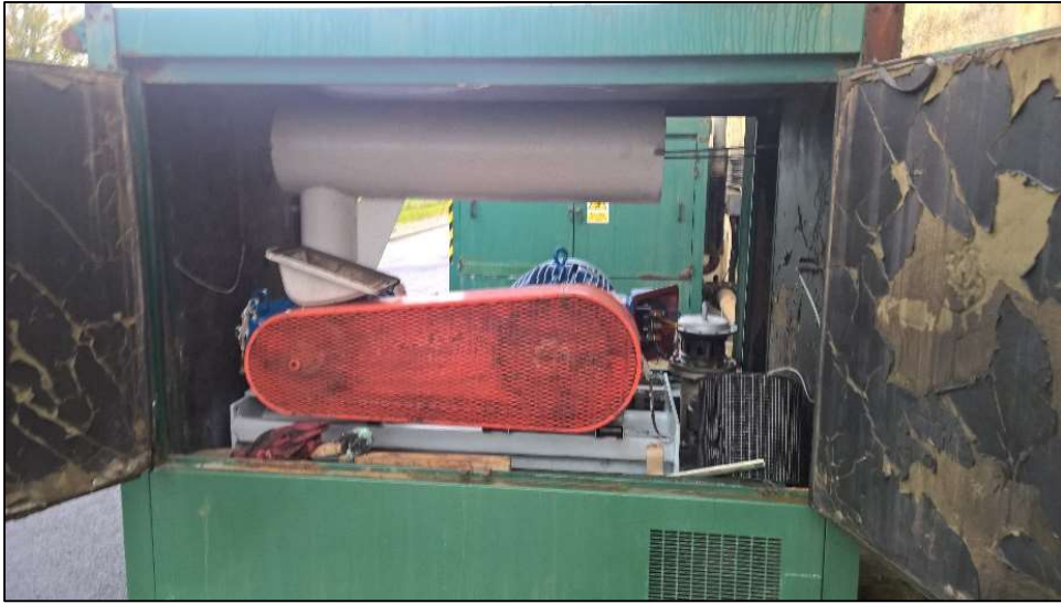
Plate 3.4.11: Air blower inside the acoustic cabinet external to the SBR
