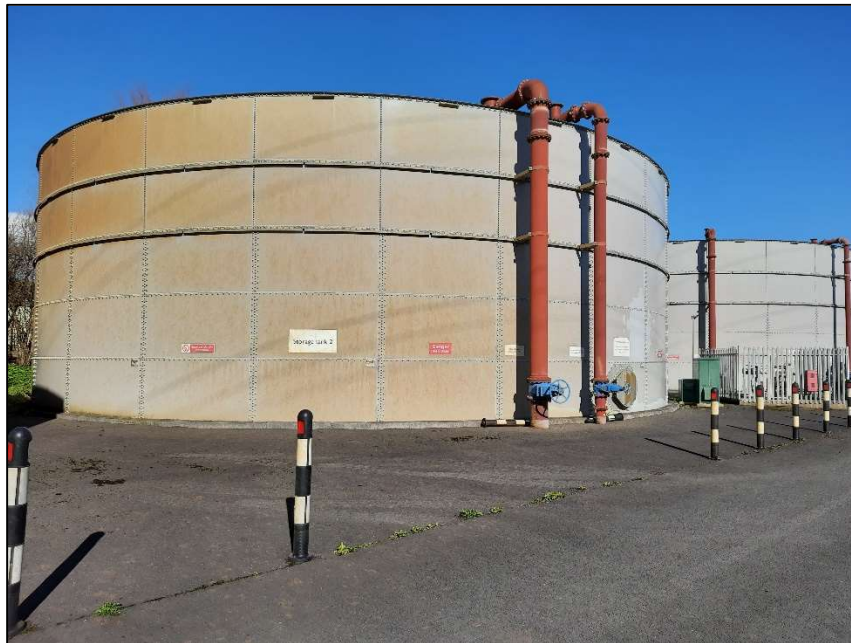
Plate 3.1.6: Completed STORs with associated pipework for leachate input
