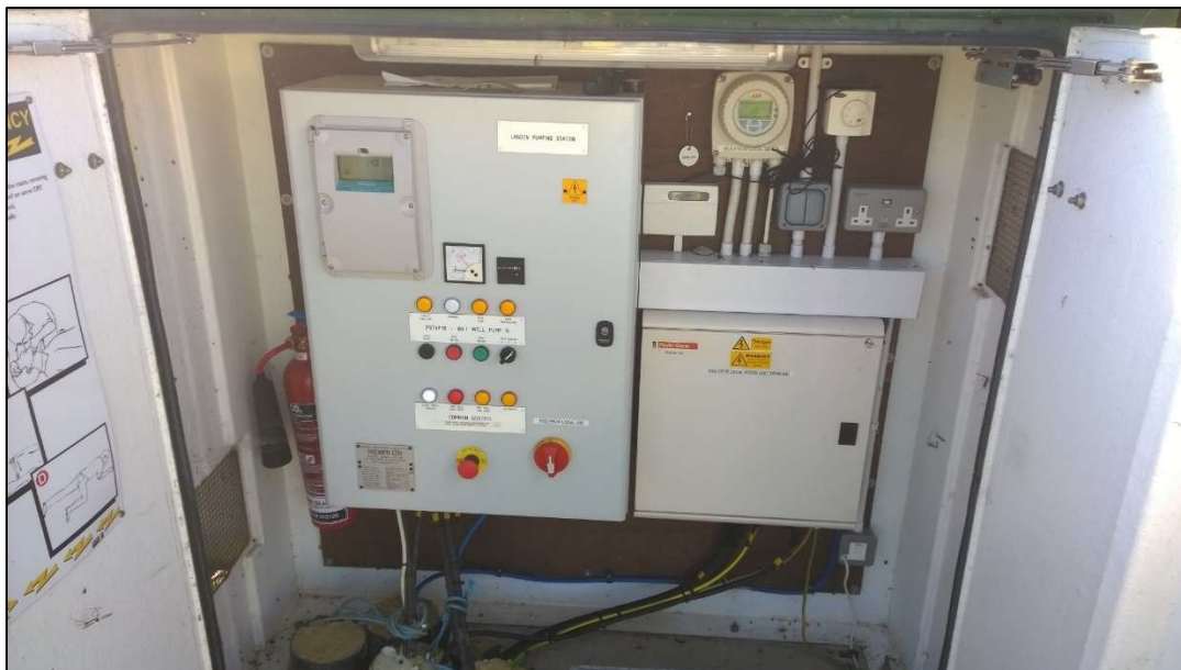
Plate 2.18: Inside the electrical housing showing the control panel serving the lagoon pumping station, August 2018
