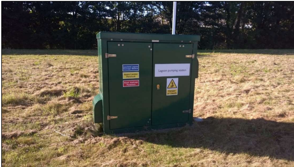
Plate 2.17: Lagoon Pumping Station (NGR SX50673 54449), Chelson Meadow Landfill 2020.
