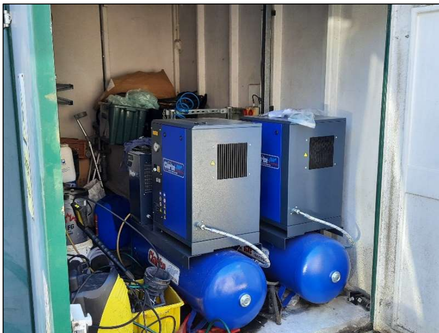
Plate 3.4.7: Clarke air compressors serving the SBR Decant Arms
