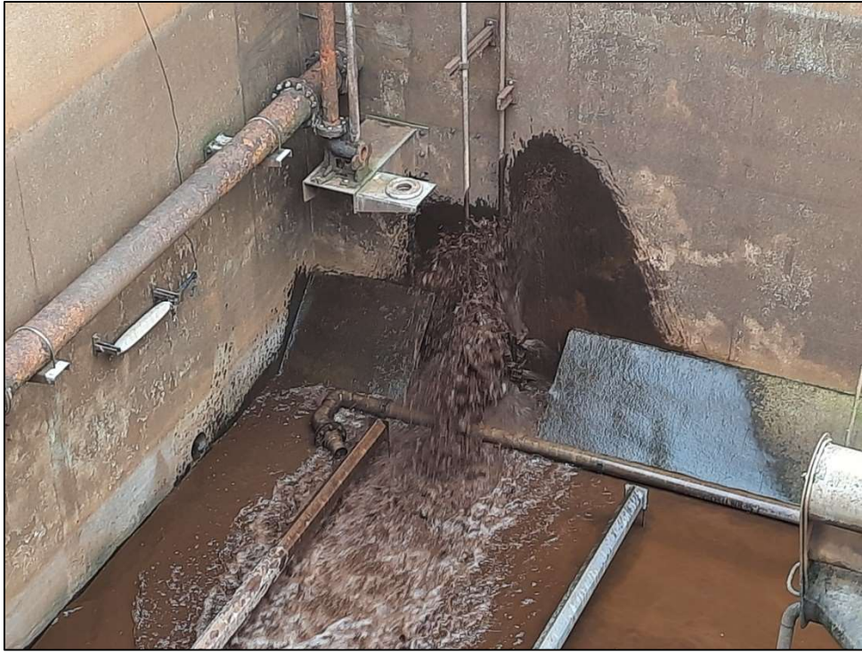
Plate 5.12: In flow of liquor into receptor SBR achieved by opening the linkage valve
