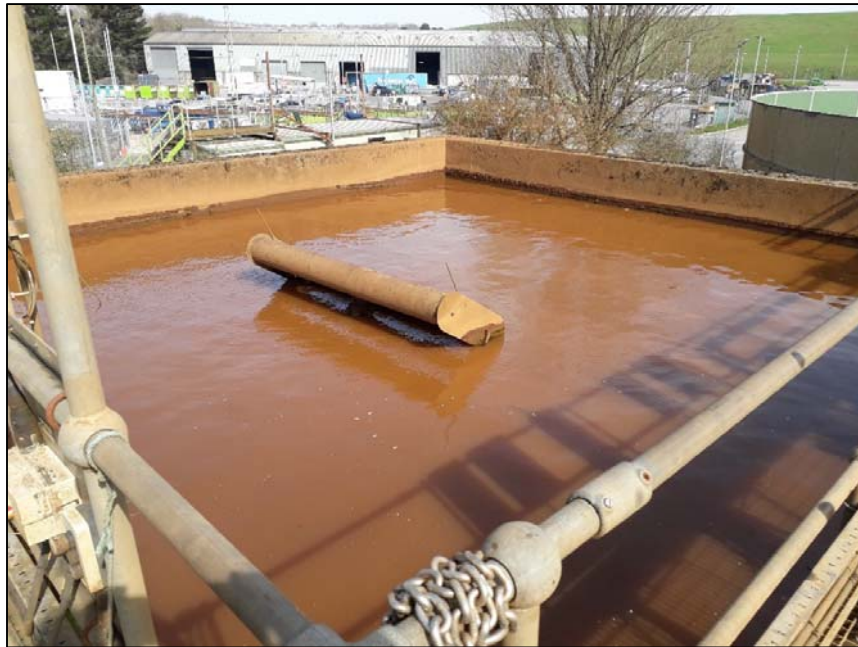
Plate 2. SBR 2 not aerating and 3hrs into its settle phase prior to discharge (PC info)
