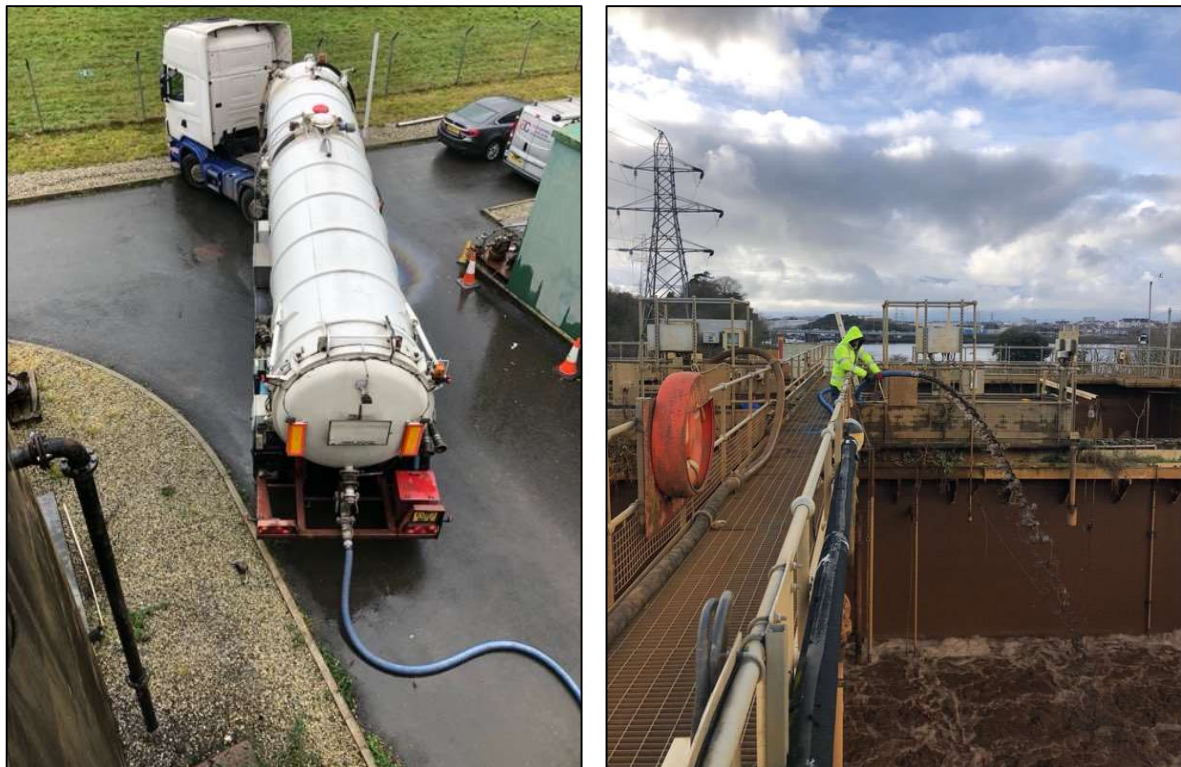
Plate 5.1: Tanker delivering activated sewage sludge to the SBR, LTP.
