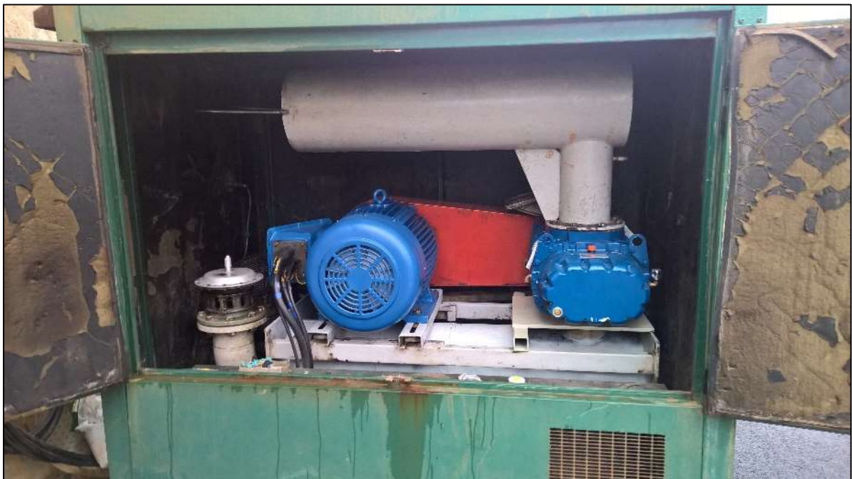
Plate 3.4.10: Air blower inside the acoustic cabinet external to the SBR
