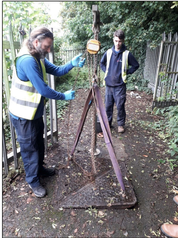
Plate 4.1.4: Ride pumping station leachate well manhole cover being lifted prior to chain test
