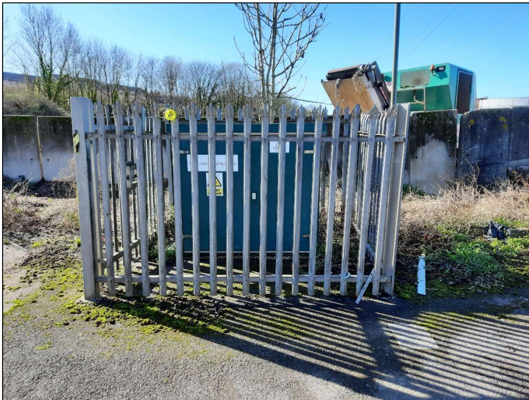
Plate 2.14: South Leat Pumping Station (NGR SX50753 54464), Chelson Meadow closed landfill 2021.
