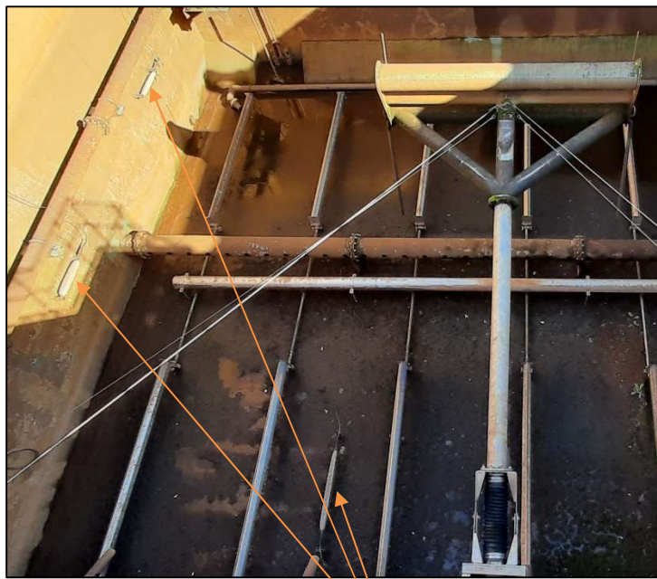
Plate 3.4.13: Sacrificial Anodes inside the SBR
