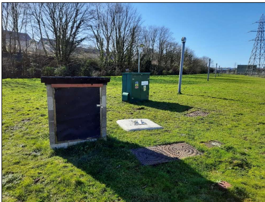
Plate 1.15: Lagoon Pumping Station, 2021
