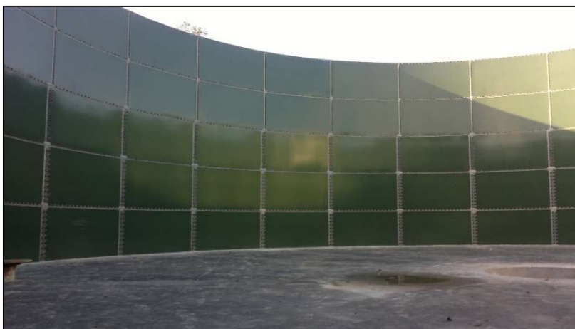
Plate 3.1.5: Internal view of glass-coated steel tank sides to STOR2
