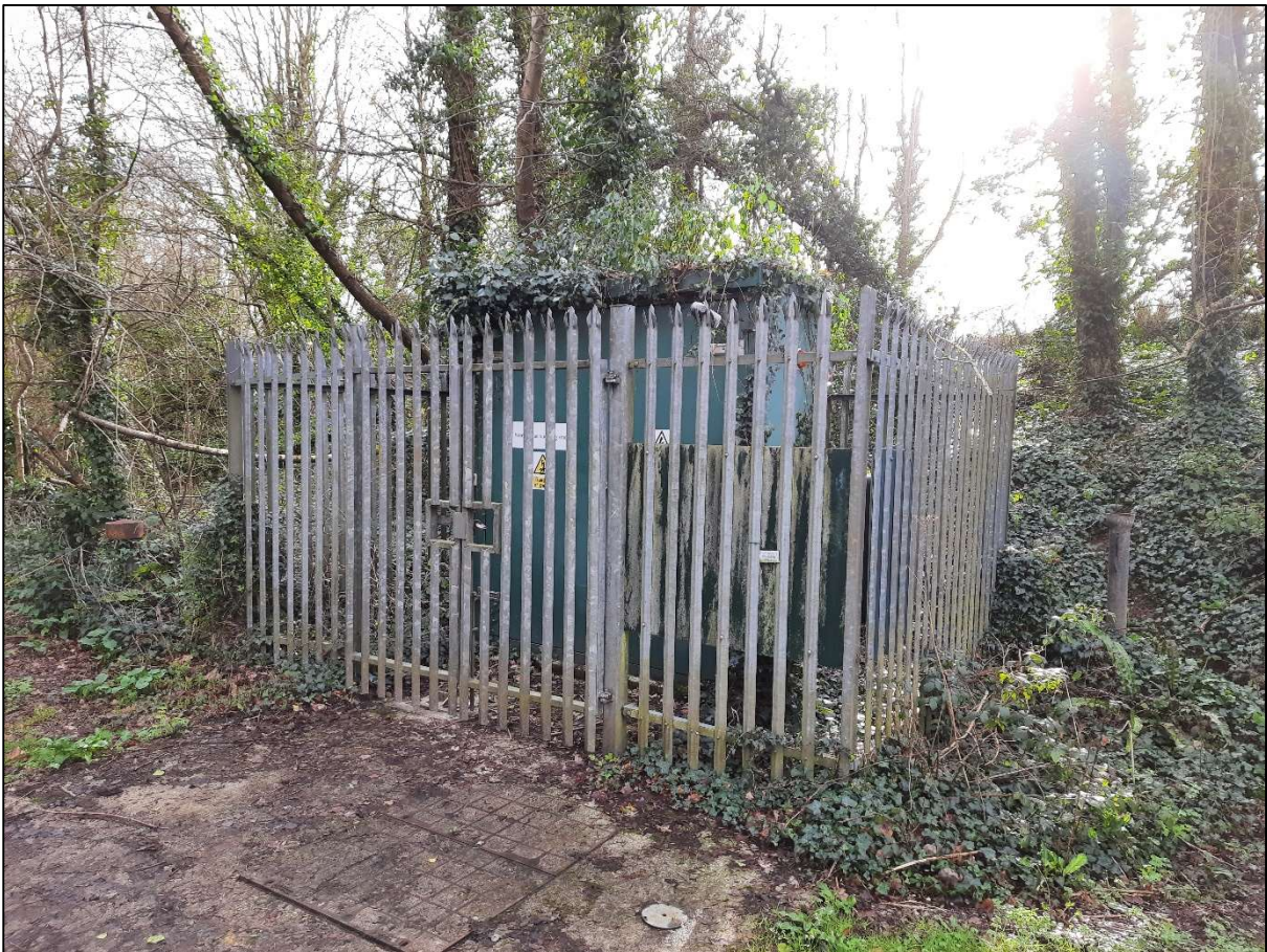
Plate 2.8: North Leat Pumping Station (NGR SX51089 55216), Chelson Meadow Closed Landfill, 2021
