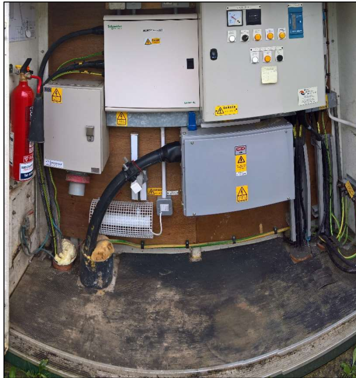
Plate 2.15: Inside the electrical housing showing the control panel serving the South Leat pumping station, August 2018
