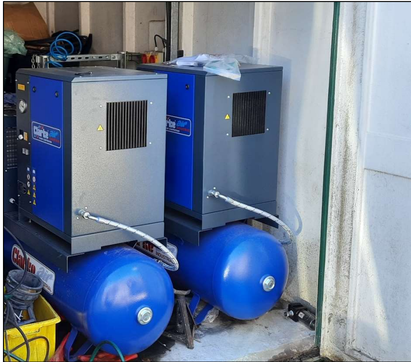
Plate 3.5.4: Washwater unit showing the two air compressors, 2021
