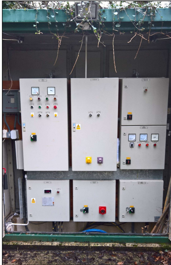
Plate 2.9: Inside the electrical housing showing the control panel serving the North Leat pumping station, August 2018
