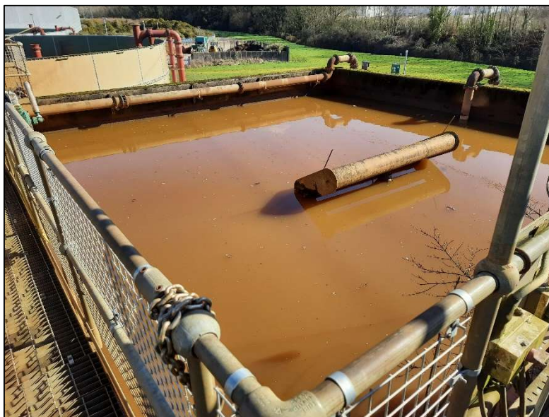
Plate 5.4: SBR in the settle phase, showing the top of the decant arm above the level of the liquor, 2021
