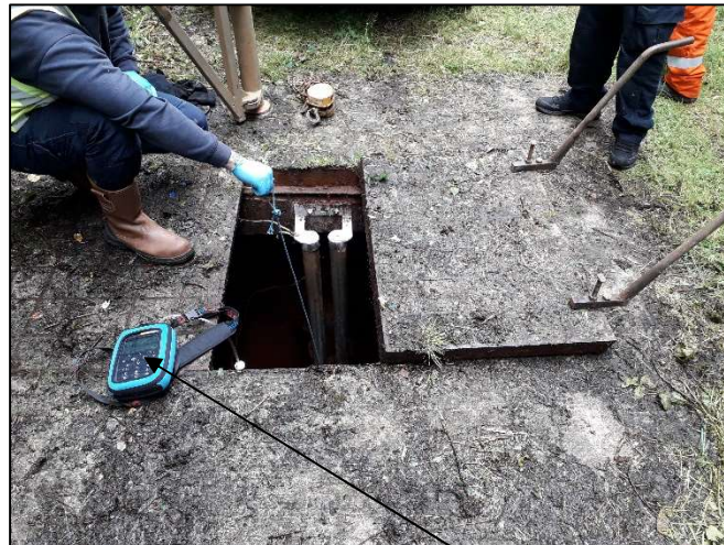
Plate 4.1.5: North leat pumping station leachate well manhole cover being removed and internal atmosphere tested for landfill gas
