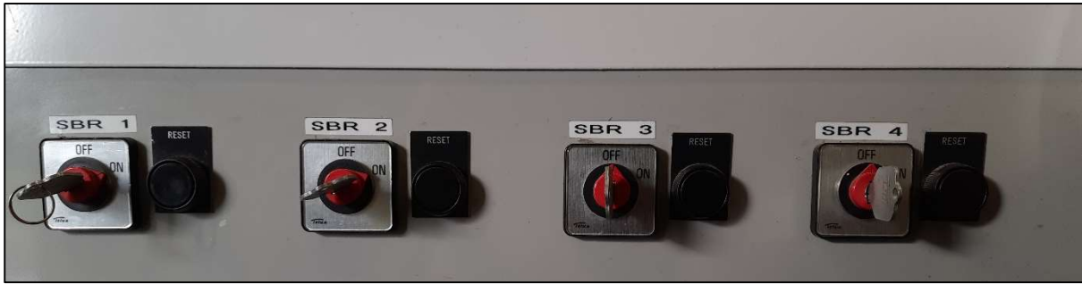
Plate 5.7: Control panel to isolate a SBRs3 & 4 from the main treatment process such that liquor can be transferred from SBR3 to SBR4
