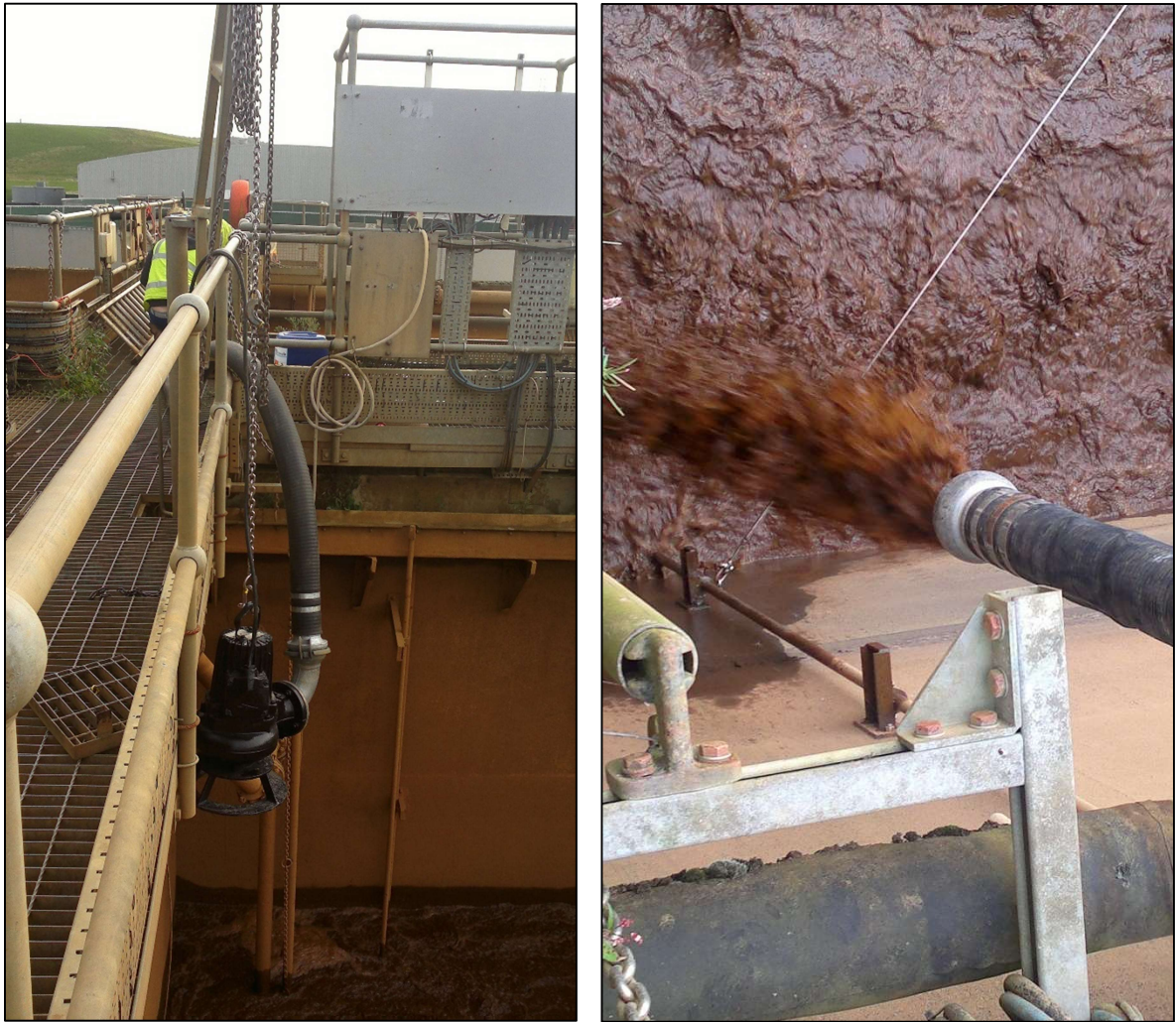
Plate 5.15: Pump being lowered into the source SBR (left) and the discharge of liquor into the receptor SBR (right)
