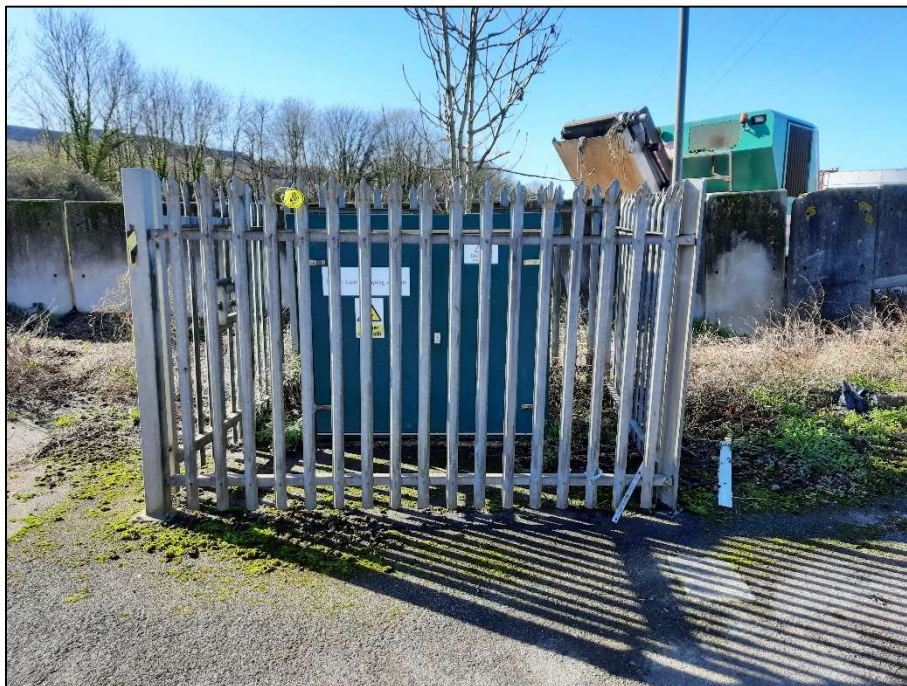
Plate 1.13: The South Leat pumping station, 2021
