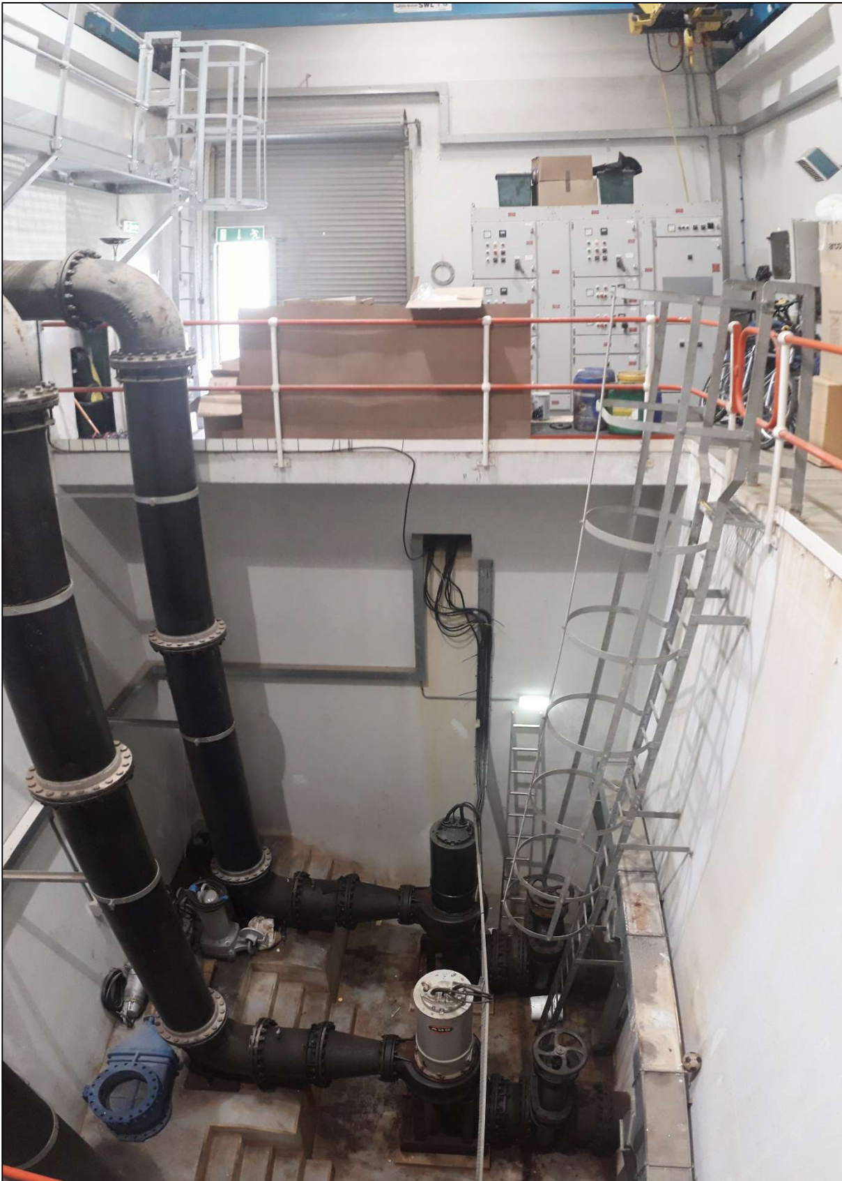
Plate 3.3.2: Internal view of PLS showing below ground pumps: ground level is at the walkway secured by railings
