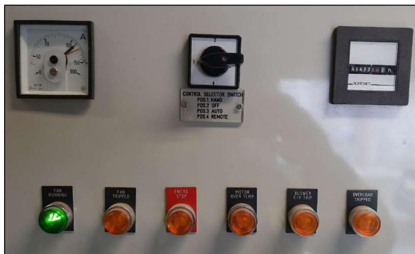
Plate 5.8: Control panel for blower 3, showing the blower has been switched to 'Hand' mode during the liquor transfer process
