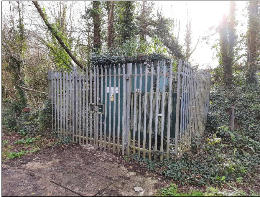
Plate 1.14: The North Leat pumping station, 2021
