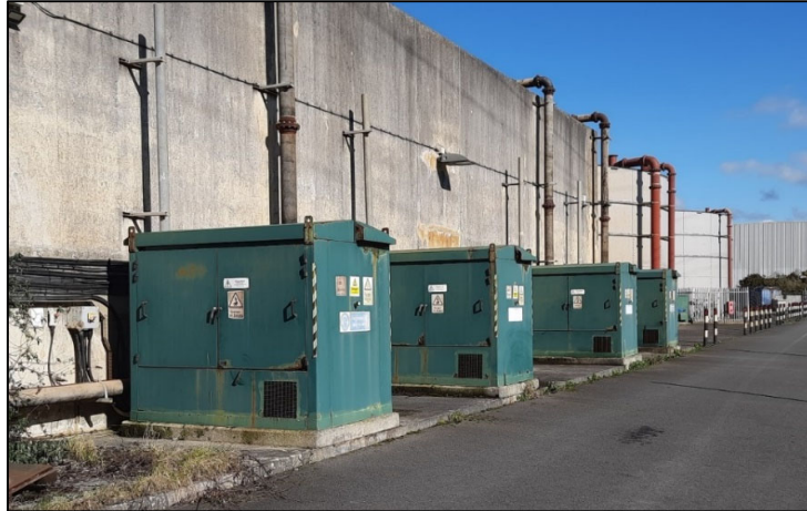
Plate 1.7: Blower cabinets alongside the SBR complex, 2021
