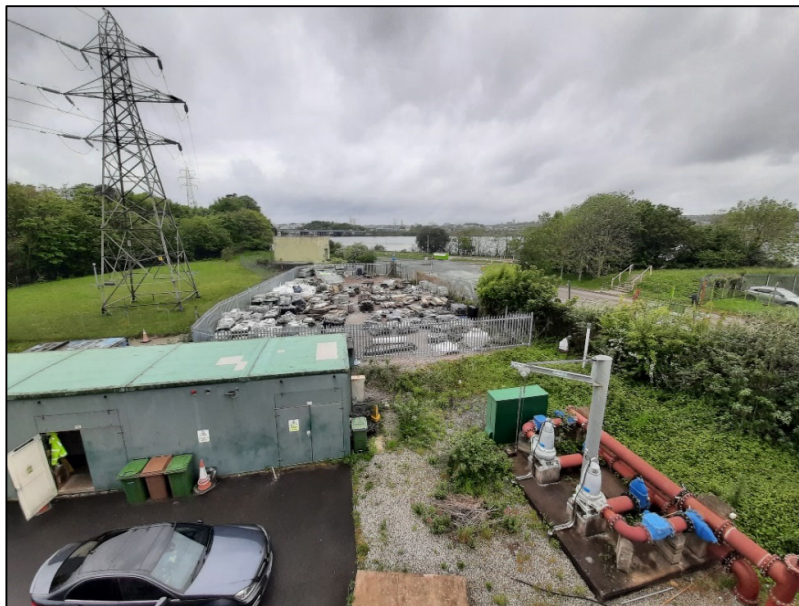
Plate 1.2: Haul road to access the LTP and the wider facility, looking west-south-west and showing the south end of the permit area, viewed from on top of the SBRs, 2021
