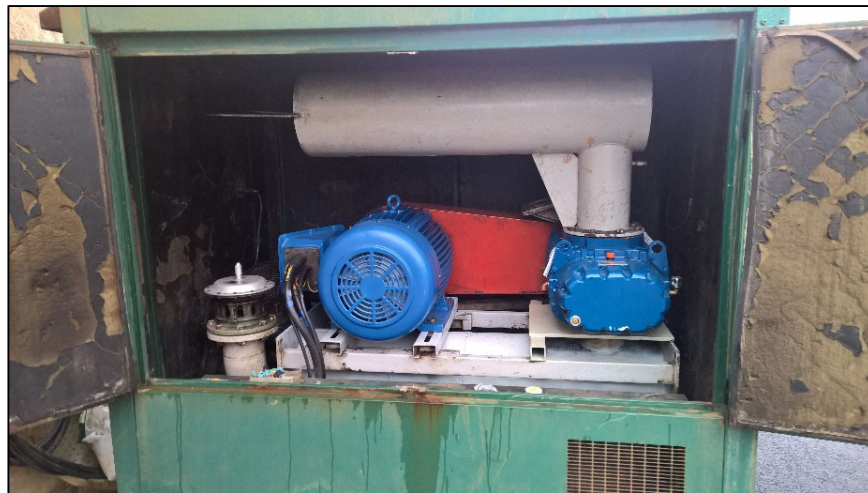
Plate 1.8: Air blower inside the acoustic cabinet external to the SBR
