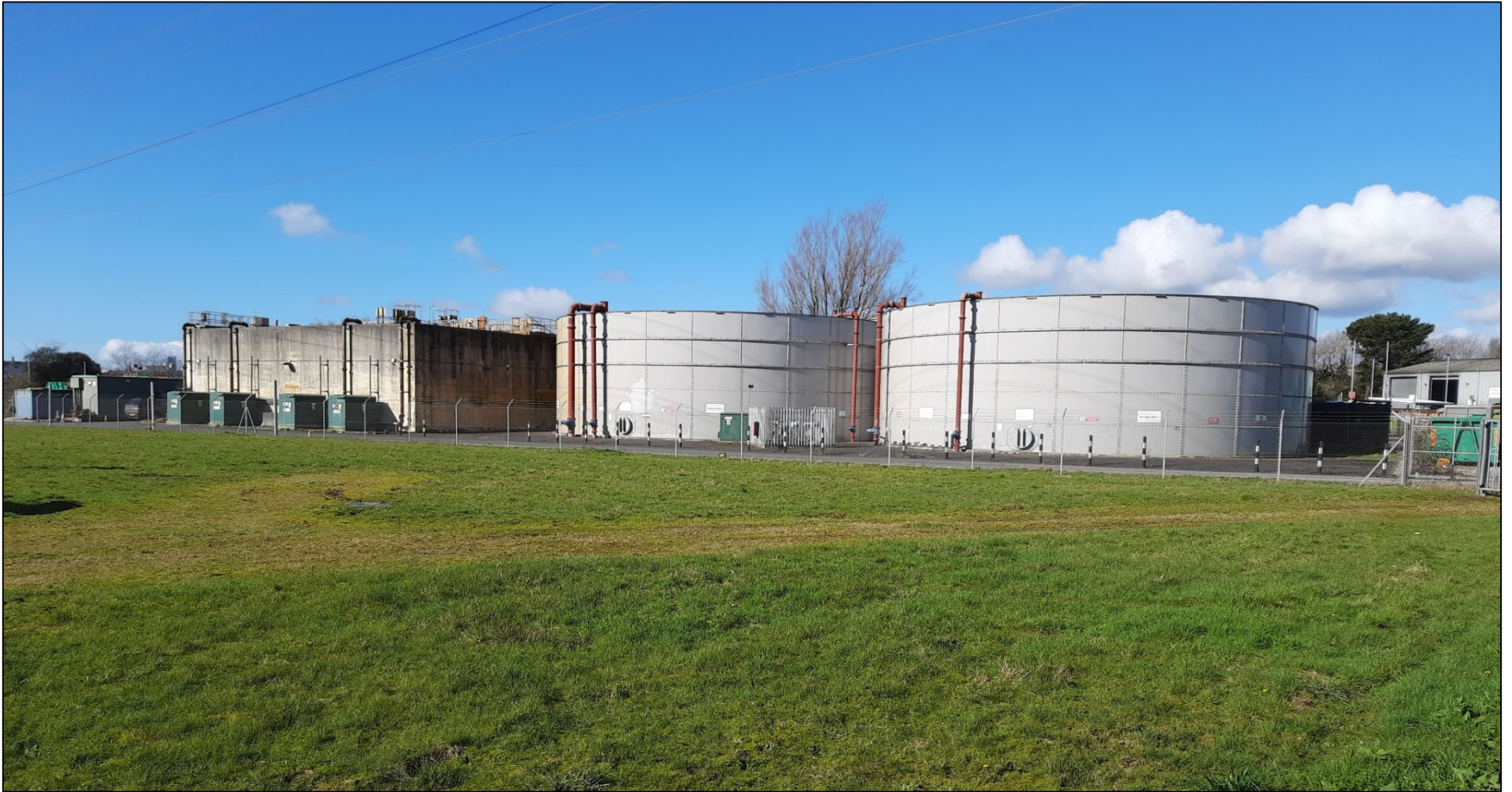
Plate 1.6: Leachate Treatment Plant, looking southwest from the lagoon pumping station, Chelson Meadow, Plymouth 2021. Infrastructure components from left to right are: Sequential Batch Reactors (SBRs), STOR 2 & STOR 1
