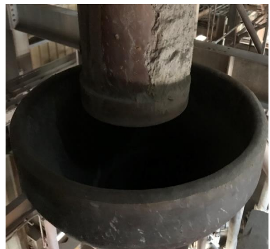
Figure 9.1 Open outlet to the underpan
