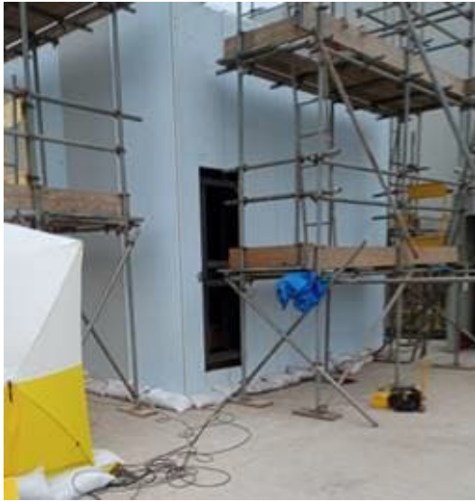
Figure 5-11 - Acoustic Enclosure with Kingspan Cladding
