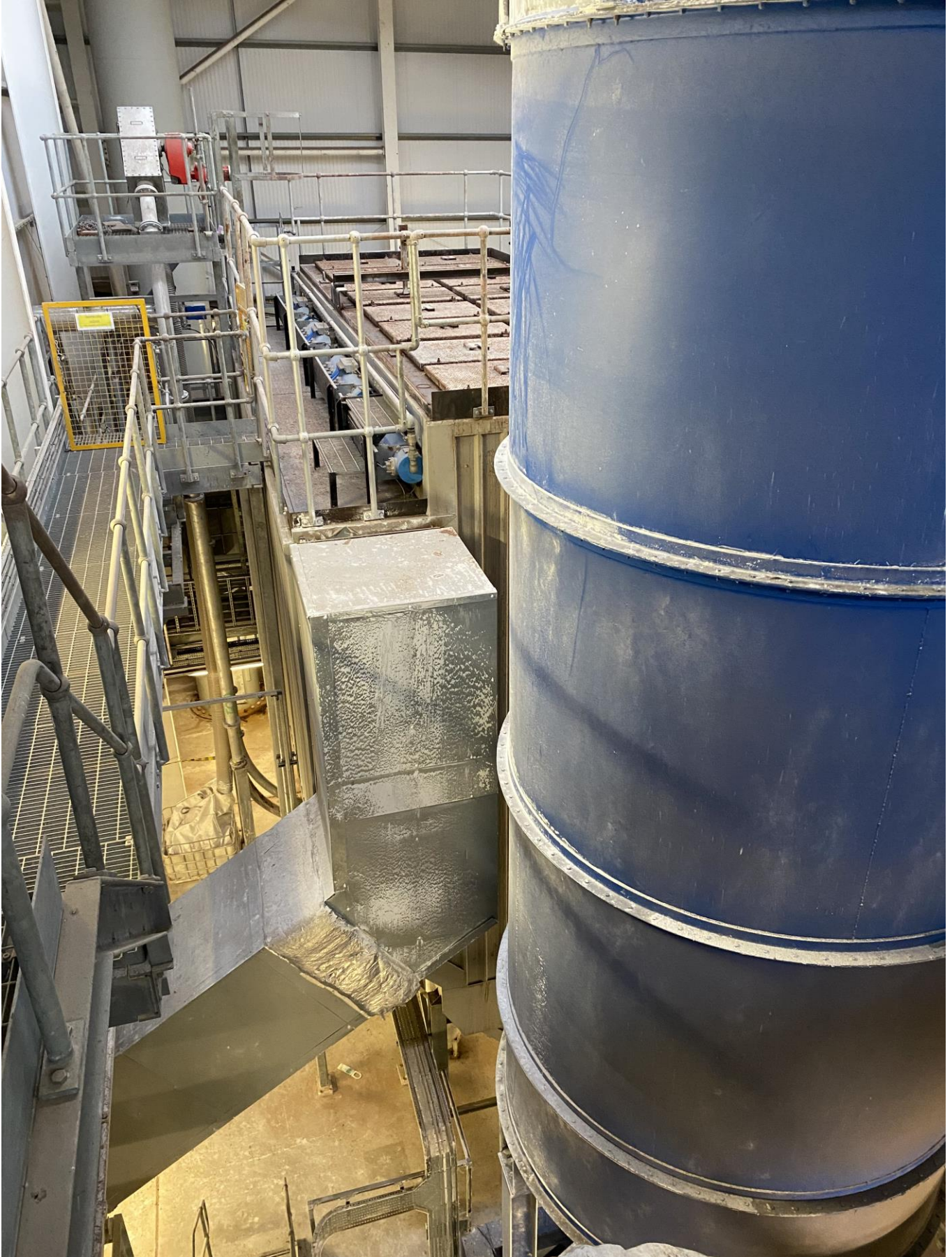
Photograph 12: Existing equipment inside processing building.
