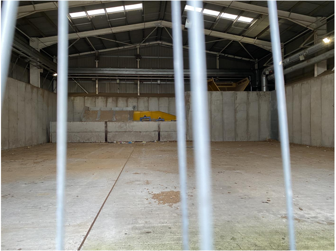
Photograph 11: Fuel reception hall.
