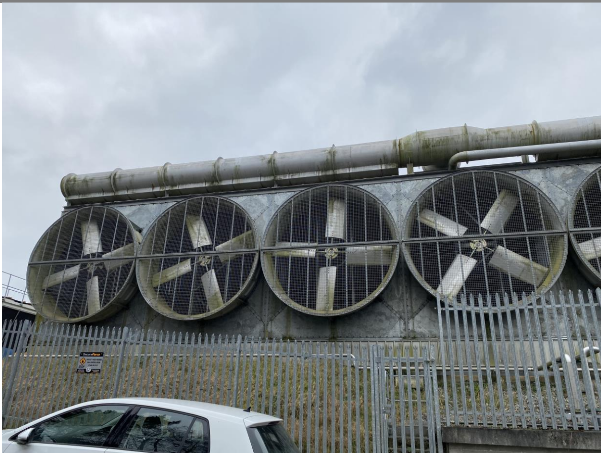
Photograph 4: Coolers at northeast end of the site.
