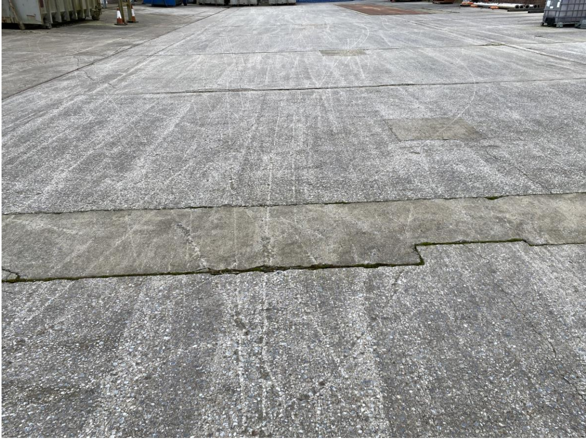
Photograph 5: Concrete pad in main yard. Existing weighbridge is visible at the top right hand side of the image.
