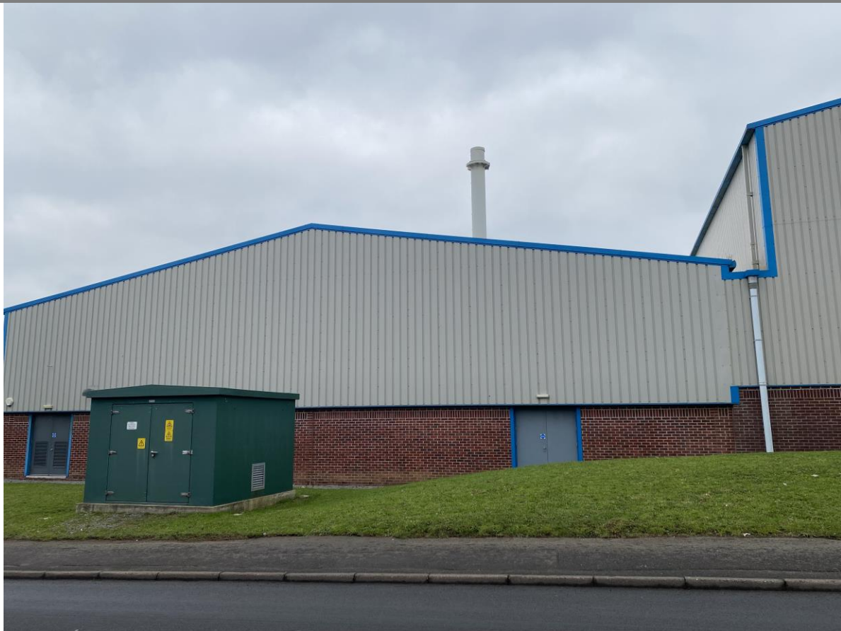
Photograph 3: Southeast façade with electricity substation in front of building and emissions stack A1 visible.
