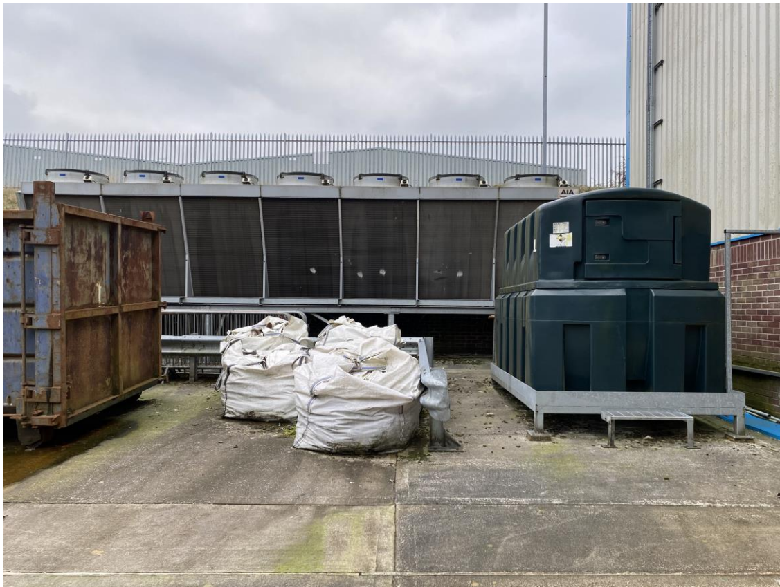
Photograph 10: Southeast corner of yard. Diesel tank on right hand side of image.
