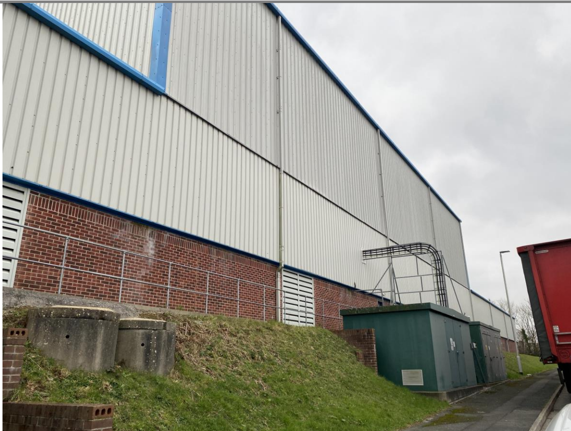
Photograph 2: Southwest façade, with electricity substations to right of image and S1 emission monitoring point to left of image.
