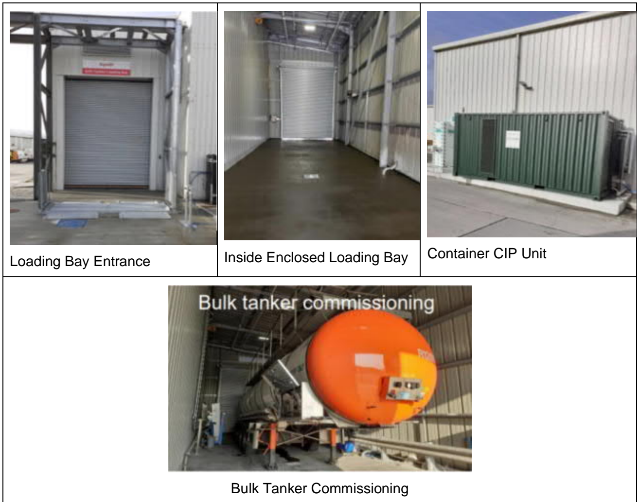
Figure 4-15 – Photographs of Installed GOS Bulk Tanker Loading Facility
