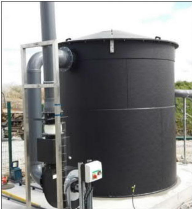
Figure 4-22 – Photograph of OCU at Contingency Lagoon
