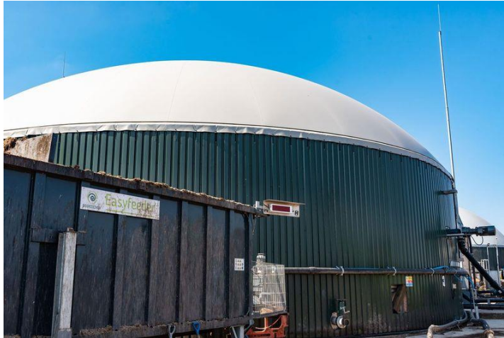
Figure 3 – Photograph of a Feeder Unit at the Site
