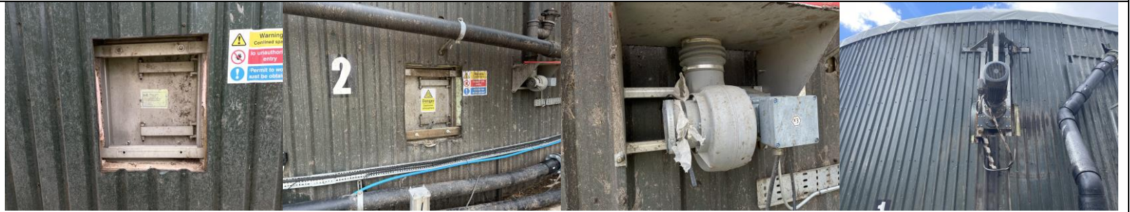
Digester access side panels and Motor encasing
