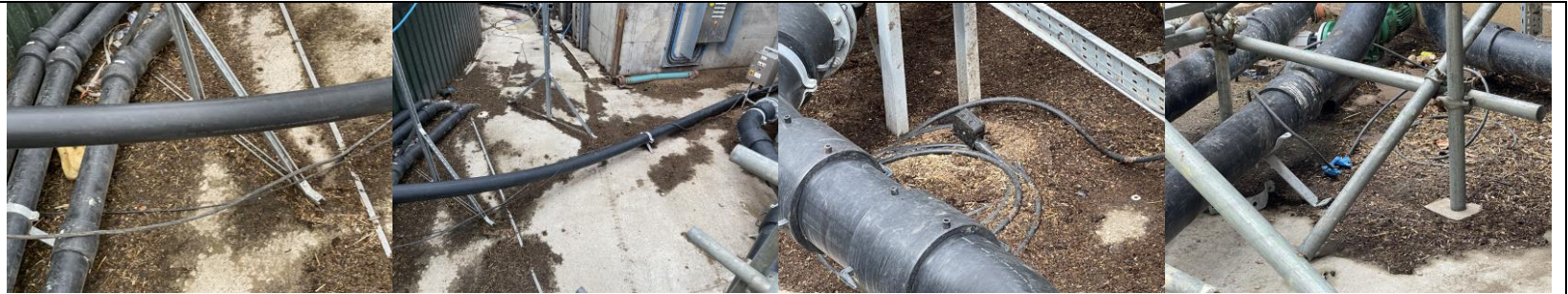
Housekeeping in yard near digestors and Slurry separation plant
