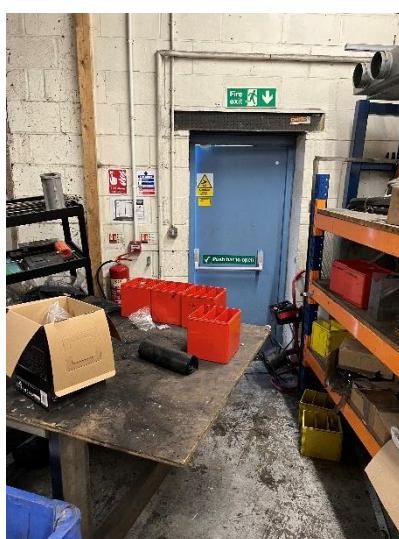
Fire exit in plant room blocked.
