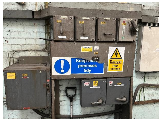
Old electrical switches need removing if not in use.
