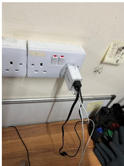
Personal electrical equipment, no PAT Tested.
