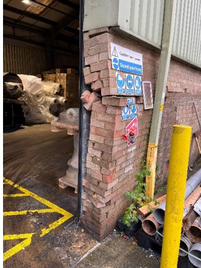
Damaged entrance wall.
