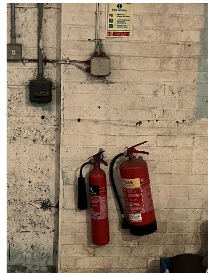
Fire extinguishers with no signage.
