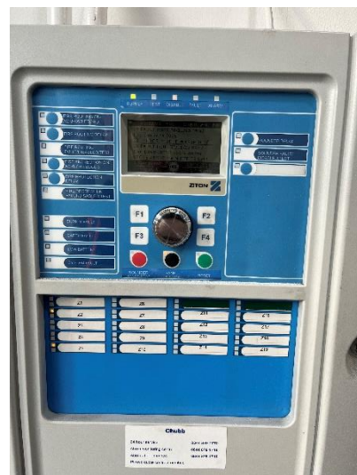
Fire Alarm showing faults.
