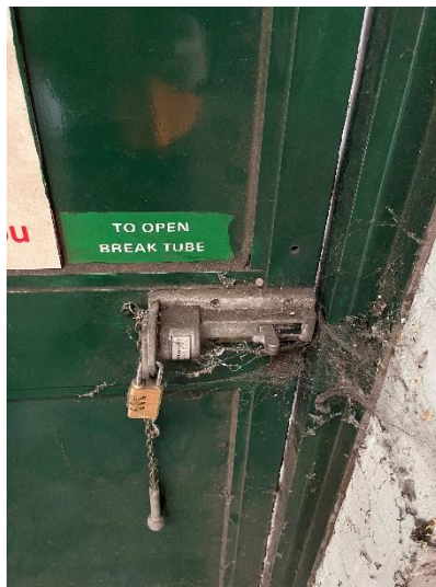
Break Glass missing, unable to secure door.
