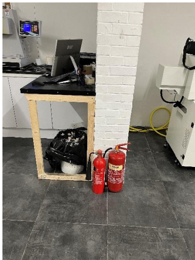
Extinguishers in QC area need fixing to the wall.
