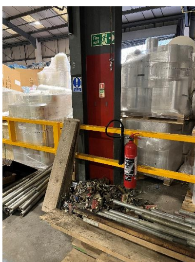
Extinguisher hard to reach.
