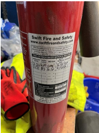
Out of date Fire Extinguisher.
