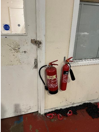
No signage for extinguishers.
