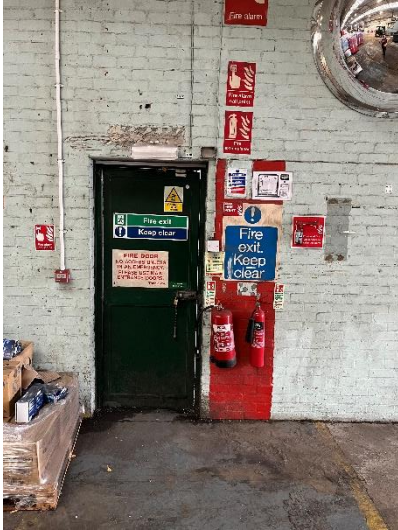
Old fire safety signage needs removing and renewing.
