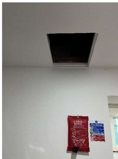
Missing hatch from office kitchen.
