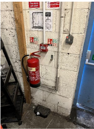
Missing fire extinguisher.
