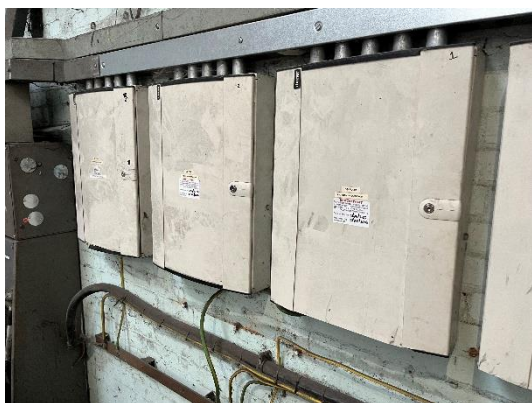
Electrical boards need signage.
