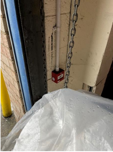
Hidden Call Point, no signage.
