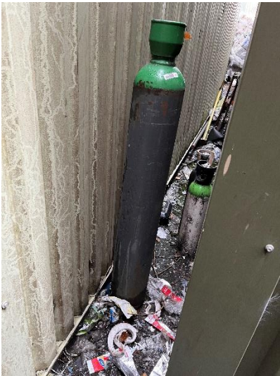
Argon cylinders at the rear, need to be removed.
