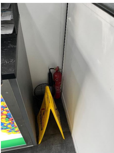
Extinguisher with pin out, in the main office.
