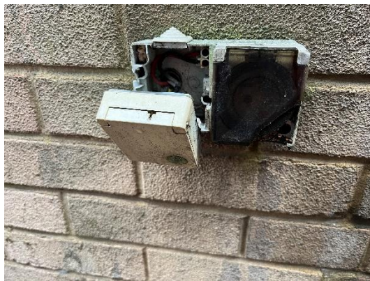
Burnt out switch at the rear.
