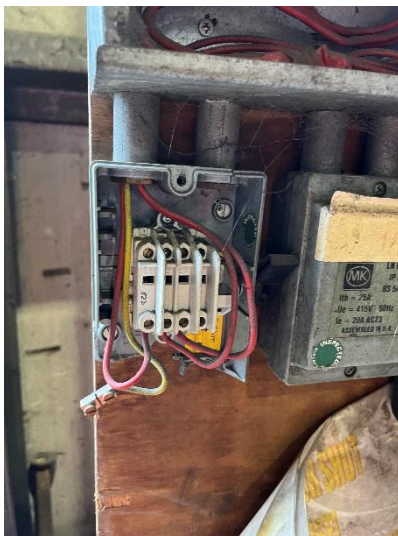
Bare electrics, needs securing.
