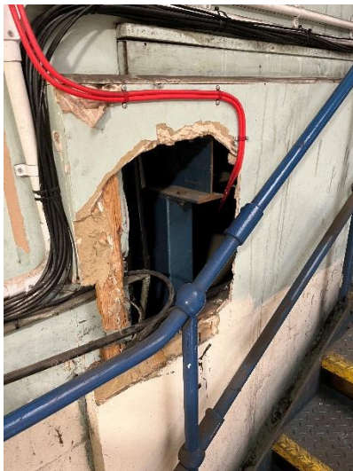
Large hole in the wall.
