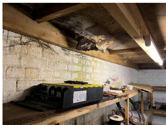
Damaged roof in stores 1st floor.
