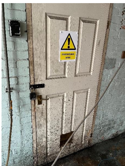
COSHH Area needs a secure door.
