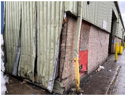
Badly damaged wall.
