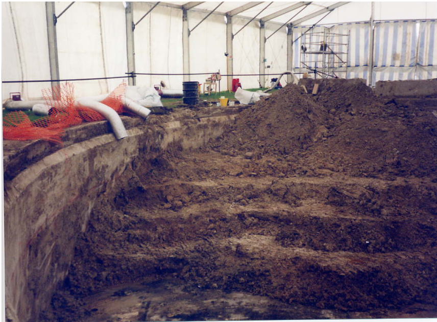
Figure 6.2. The Catapult Pit during excavation. Note the waste was excavated in layers and benched for safety purposes.
