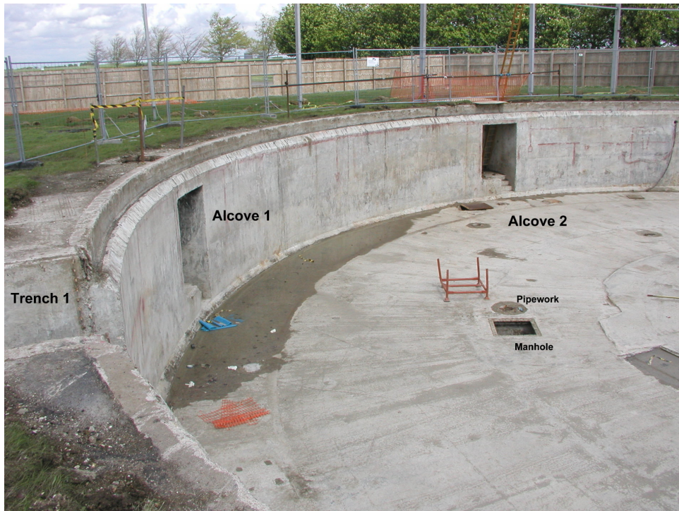
Figure 4.2. The Catapult Pit interior. Note the additional features: Alcove 1 and 2, manhole and pipework.
