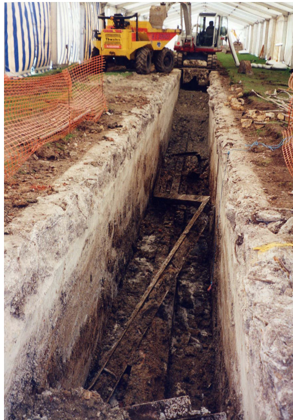
Figure 6.3. Excavations in the Trench. Note the small excavator in the distance straddling the trench and loading waste into a dumper.
