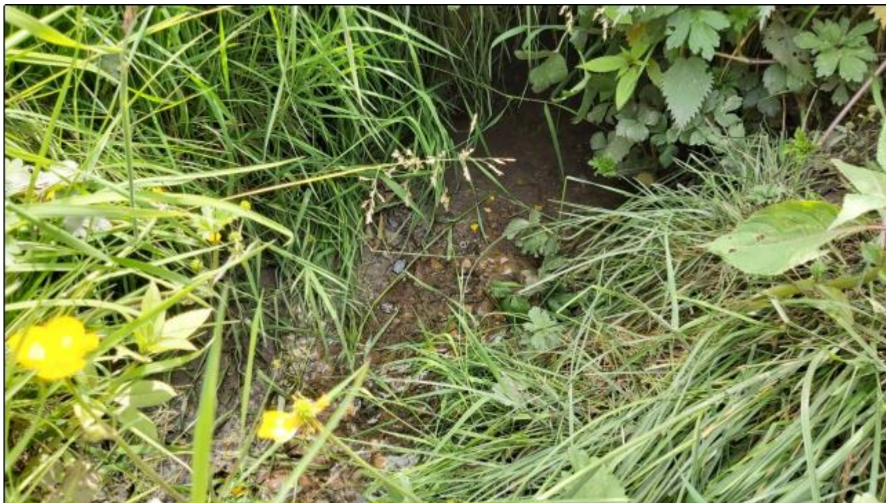
Hey Head Drain - Water Present but negligible apparent flow
