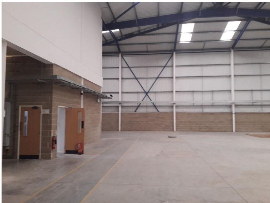
Photograph showing the western half of the building with associated internal offices.
