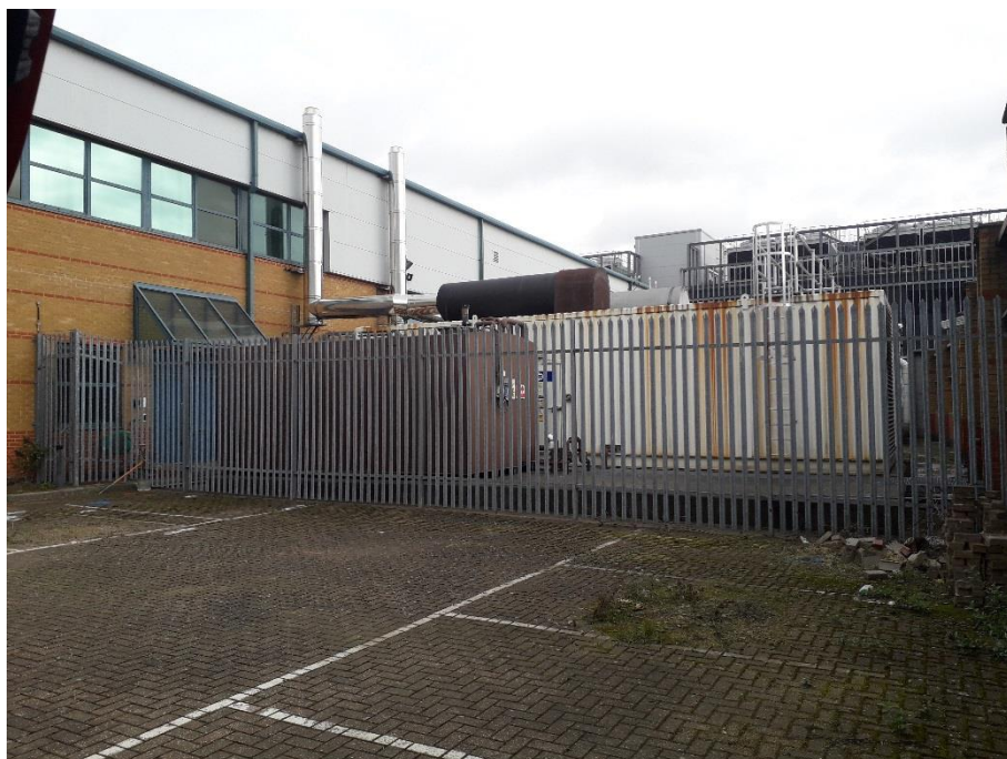
Photograph looking north east towards the adjacent part of the building and the current external slabs with associated generators etc.
