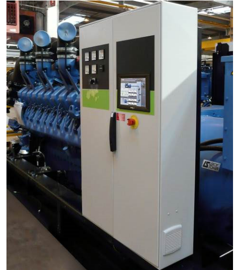
Embedded cabinet APM802 on genset.
