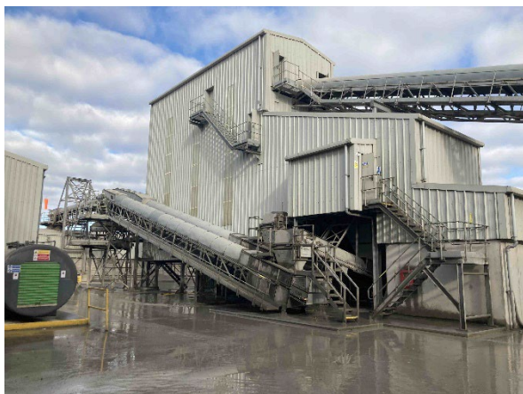
Example of covered conveyors
