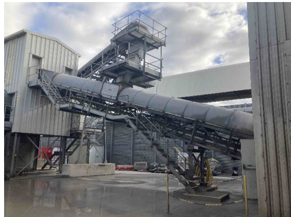
Example of covered conveyor
