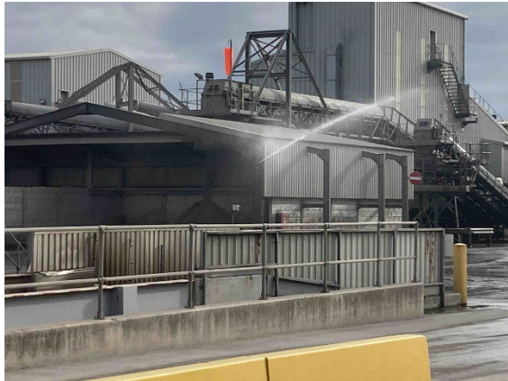
Example of external sprinkler
