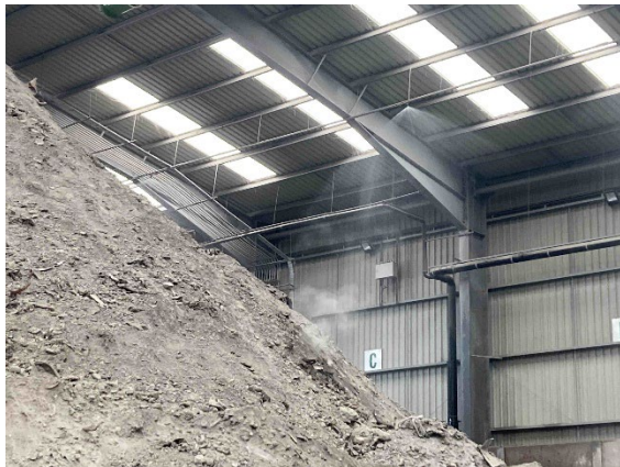
View of internal sprinkler in IBA reception area
