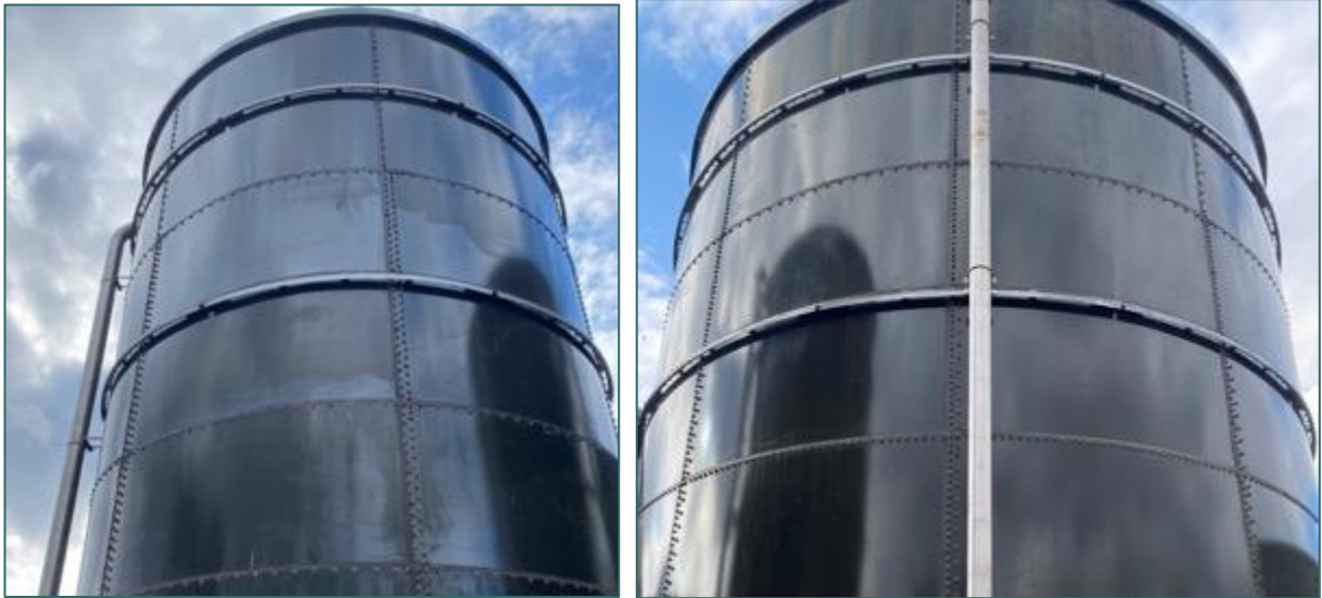
Image 1: New Glass Coated Steel Waste Storage Tanks
