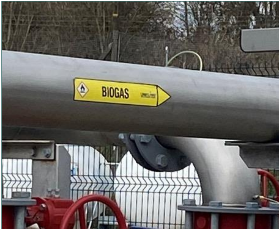
Image 5: Pipeline Labelling to Show Contents and Flow Direction
