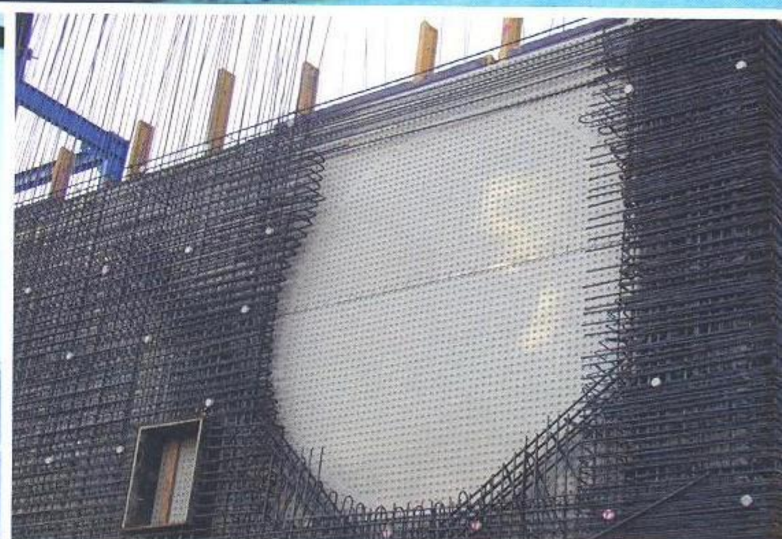
Steuler also installs Bekaplast™ as concrete scrubber linings in flue gas desulphurisation plants.
