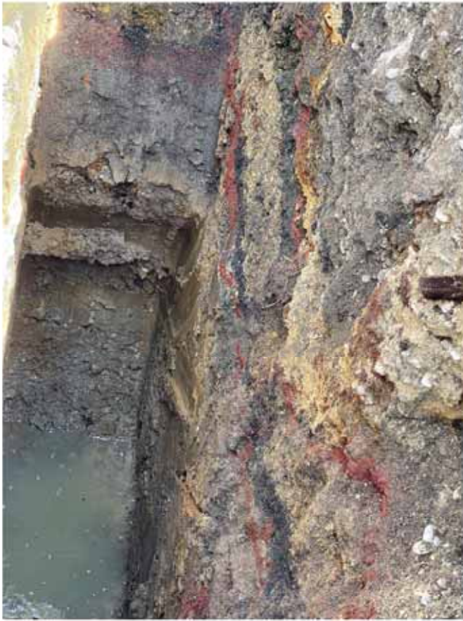
4. Side backwall and groundwater
