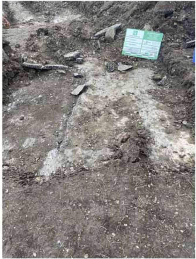
2. Concrete obstruction in excavation
